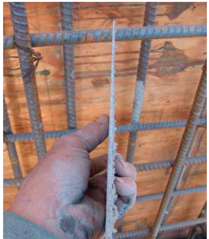
Fig. 4: Removed sample of initial shotcrete placement
