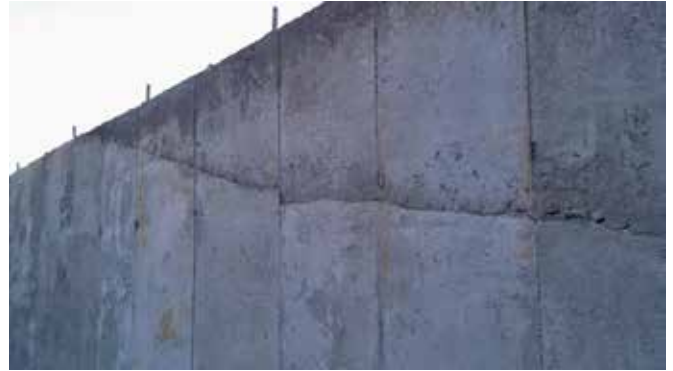
Fig. 1: Prominent cold joint in a form-and-pour wall
