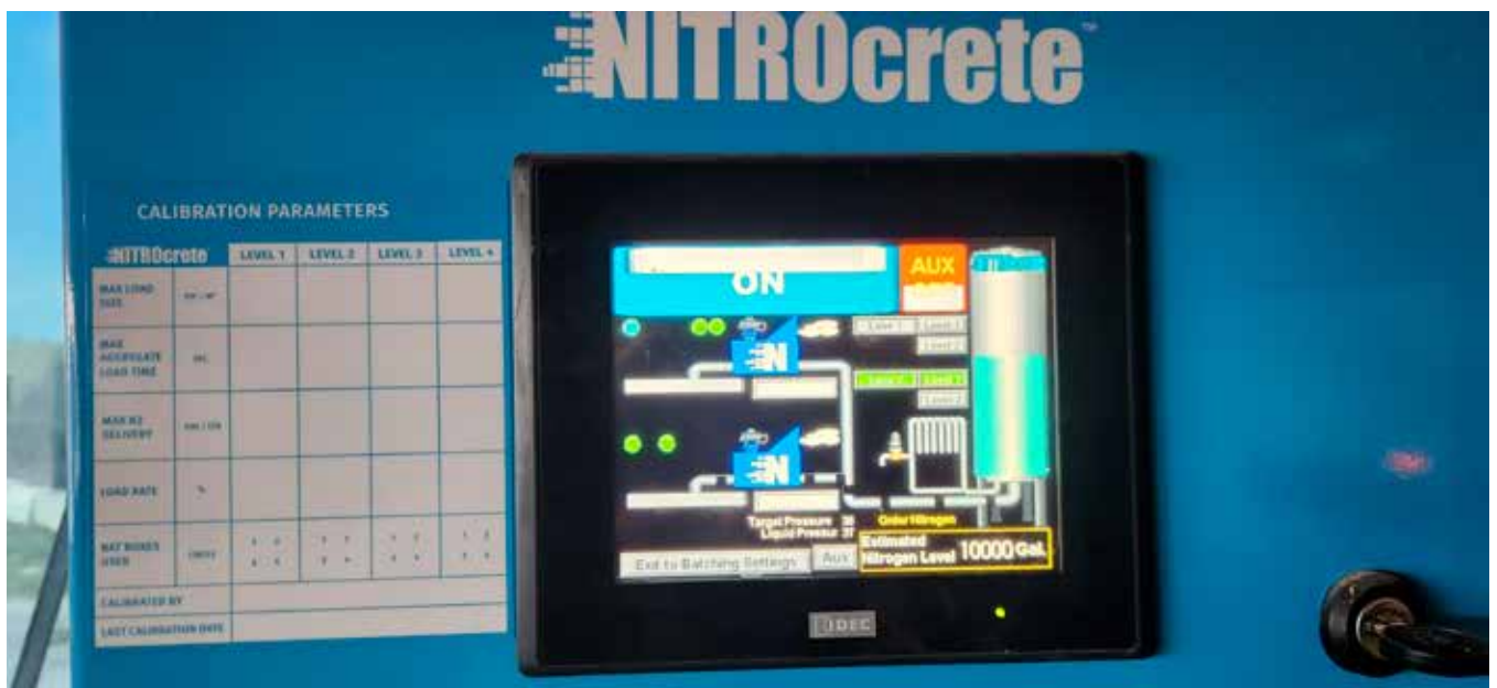
Fig. 5: Automated aggregate cooling systems integrated into batch plant operations
