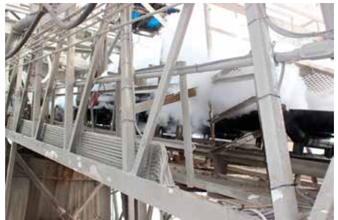
Fig. 3: Dispensing heads apply the liquid nitrogen to the warm aggregates
