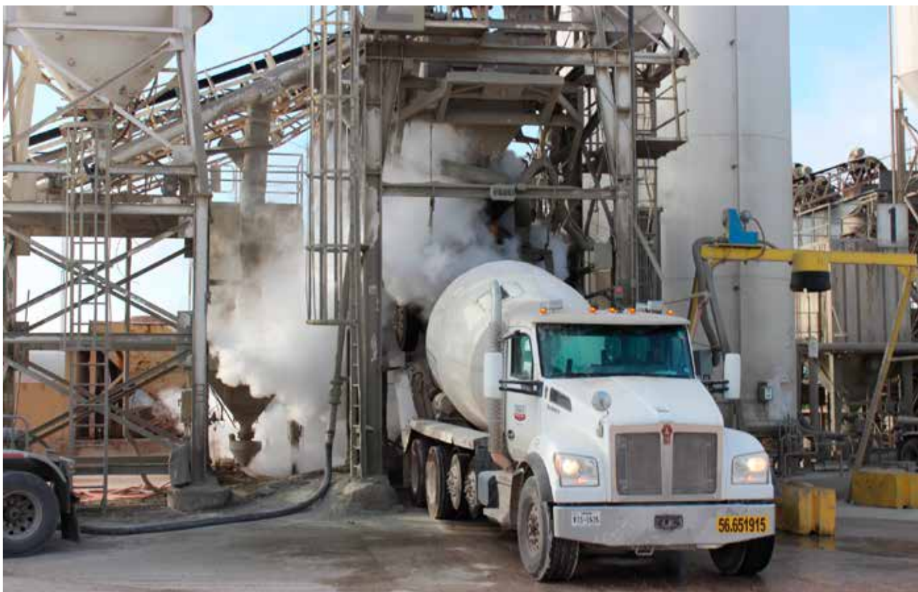
Fig. 1: Ready-mix truck being loaded with cooled aggregates via a NITROcrete liquid nitrogen cooling system
