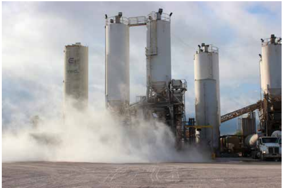
Fig. 2: Insulated cryogenic liquid nitrogen storage tank
