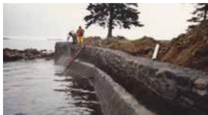
Fig. 4: While working with the 8 ft (2.4 m) tides at various levels the shotcrete placement begins from bottom to top and over the wall down the backside to the newly installed filter fabric and crushed stone backside drainage feature to capture and safely remove the overwash drainage from extreme tides
