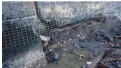
Fig. 3: The same procedure as in #1 was all in preparation of the dry-mix shotcrete placement at various thickness to provide a reasonable looking non troweled finish
