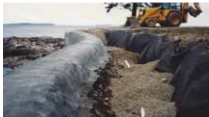
Fig. 2: The final stages of completing the backside drain system up to the top of the seawall
