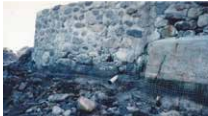
Fig. 1: Cleaning the bottom of the seawall at low tide by fresh water blasting and securing a new "through drains" and placement of new galvanized 2 x 2 WWF, tied to epoxy set 6 in. galvanized anchor bolts on a 2 ft x 2 ft pattern
