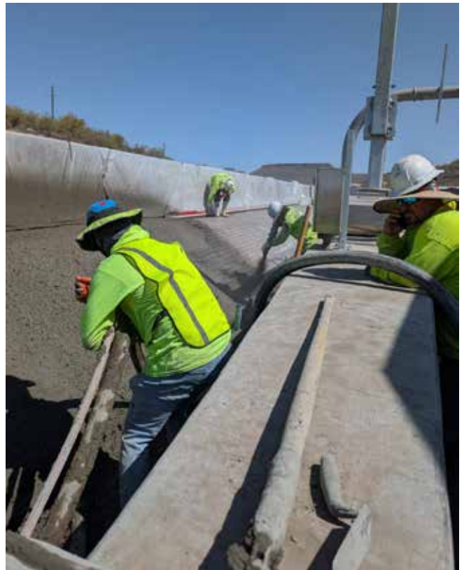
Fig. 3: Shotcrete crew placing concrete on reinforced slope protection along a highway embankment in Arizona
