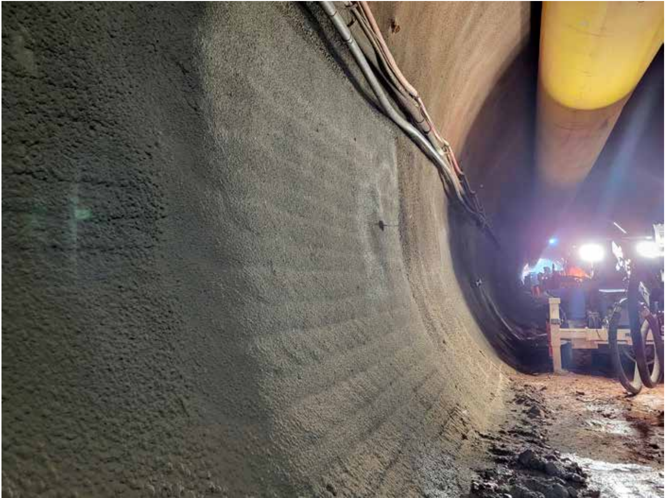
Fig. 5: A sprayed area with good concrete quality; the pattern is still visible, but significantly less pronounced
