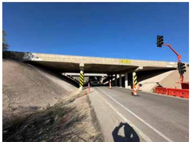
Fig. 6: Completed shotcrete slope protection under a highway overpass for long-term erosion control and durability
