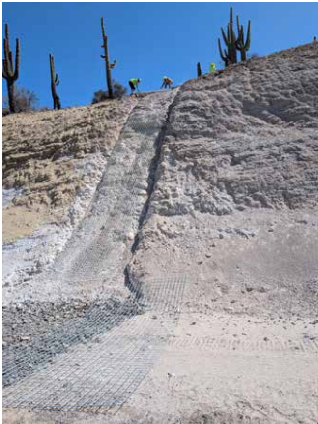
Fig. 2: Rebar installation on a steep slope for the upcoming shotcrete application and erosion control system
