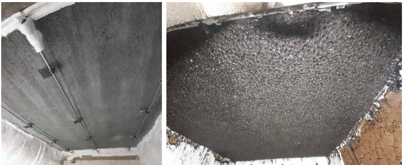
Fig. 8: HCM testing panel before (LEFT) and after (RIGHT) being exposed to 2372°F (1300°C) for 180 minutes. No visible damage was reported after testing. Photo credit: CERIB (2023).
