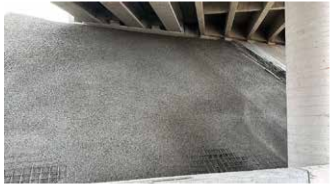
Fig. 5: Finished shotcrete wall with uniform texture and proper compaction for structural slope stabilization
