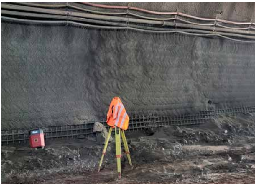
Fig. 4: The appearance of sprayed surfaces when the shotcrete mixture is too fluid; a clearly visible pattern can be observed, which is often undesirable
