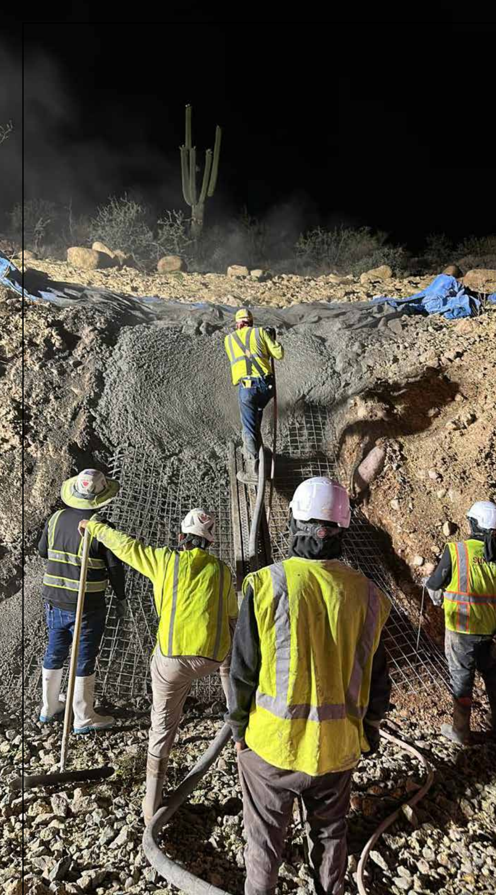
Fig. 4: Shotcrete crew applying concrete over rebar for wash lining and slope stabilization in desert terrain
