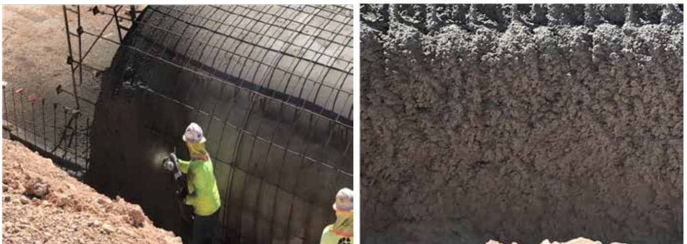
Fig. 8: Wrong angle shooting results in surface waviness
