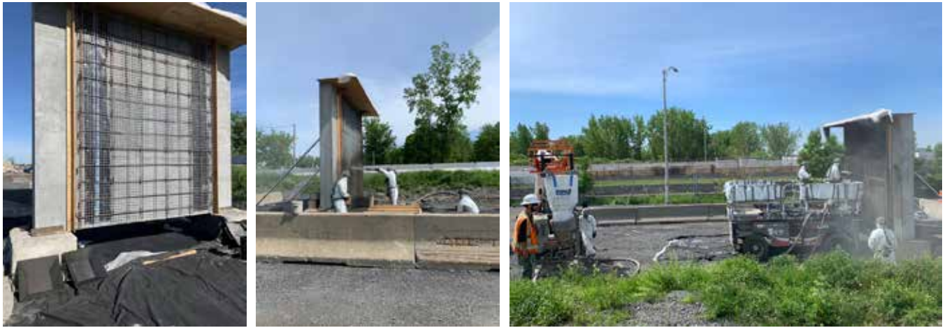
Fig. 7: Preparation of the panel with dry-mix shotcrete King® MS-D1 FSR for the HCM fire curve testing by the contractor Groupe LB. Photo credit: Sika Canada (2022).
