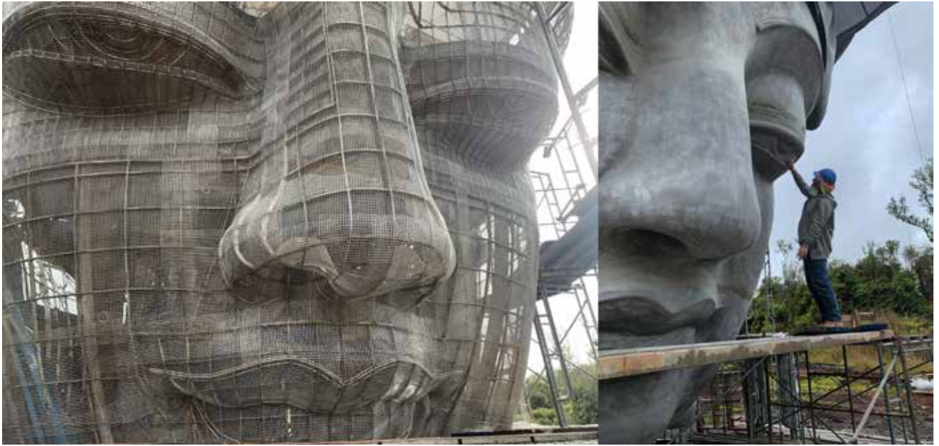
Fig. 5: Armature with mesh and 0.375 in. steel rods for better definition and finished mortar layer
