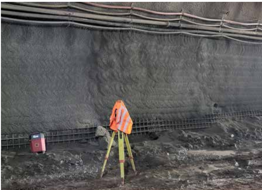
Fig. 4: The appearance of sprayed surfaces when the shotcrete mixture is too fluid; a clearly visible pattern can be observed, which is often undesirable
