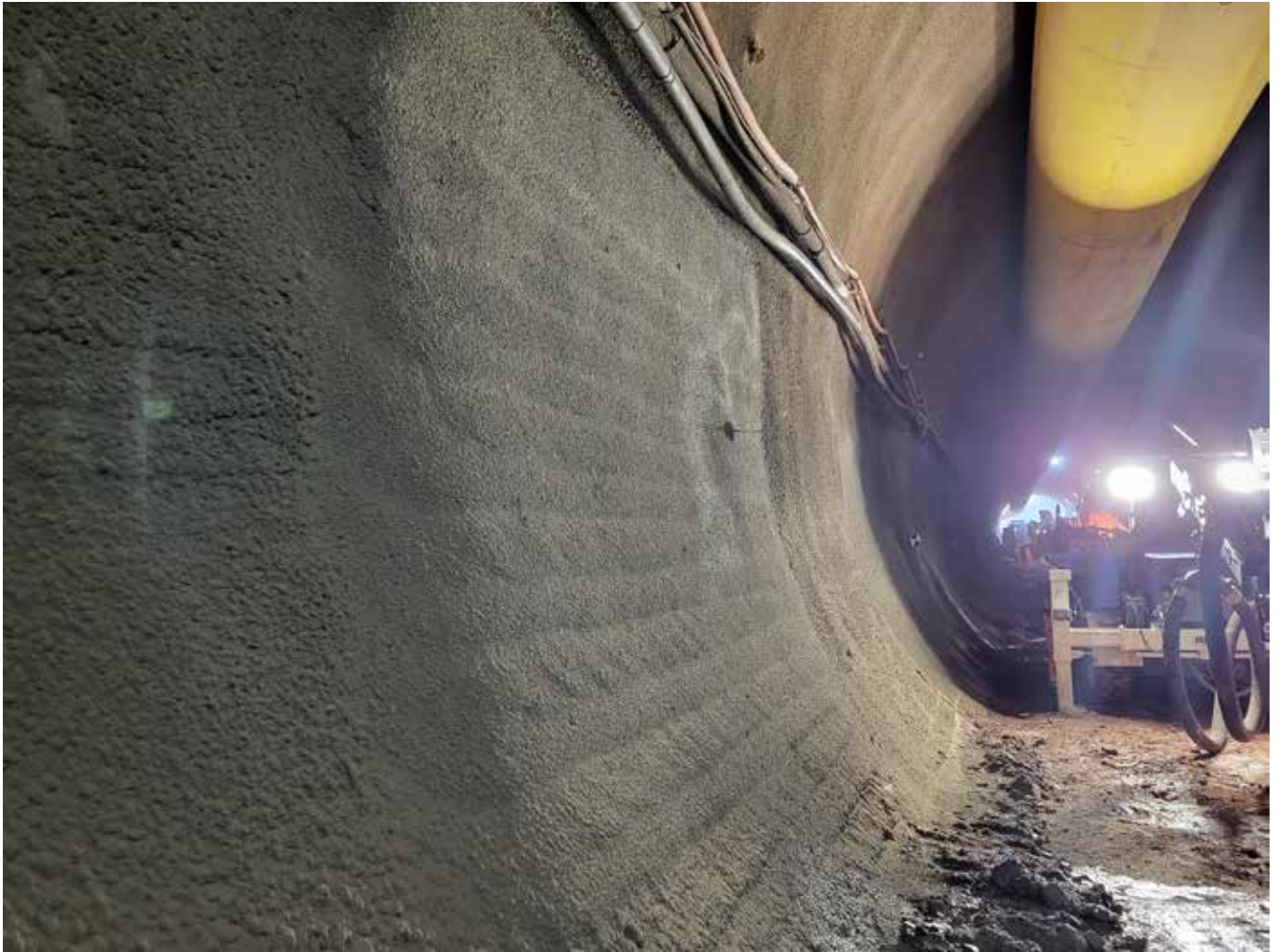
Fig. 5: A sprayed area with good concrete quality; the pattern is still visible, but significantly less pronounced
