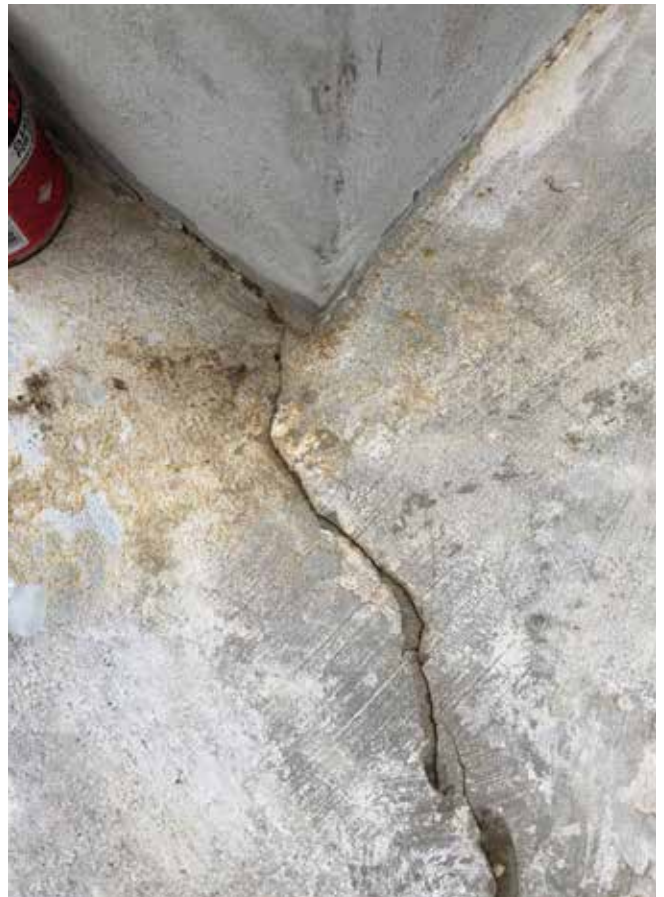
Fig. 2: Shrinkage crack worsened by freeze-thaw cycling.
