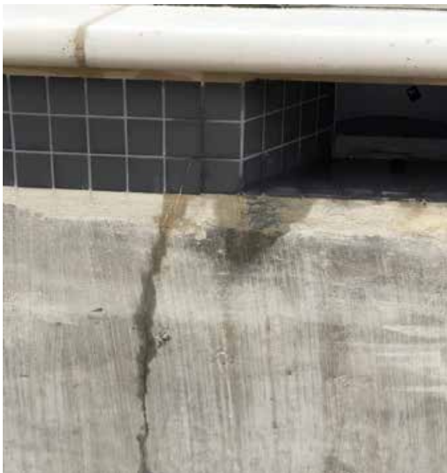
Fig. 7: Shrinkage crack at skimmer throat.
