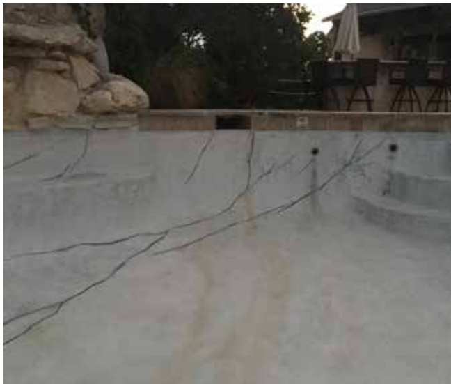
Fig. 1: Cracks due to heavy rock structure and subgrade settlement.
