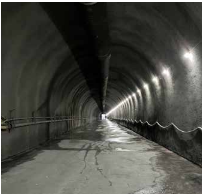
Smoothing shotcrete interior surface complete looking out of tunnel toward the portal
