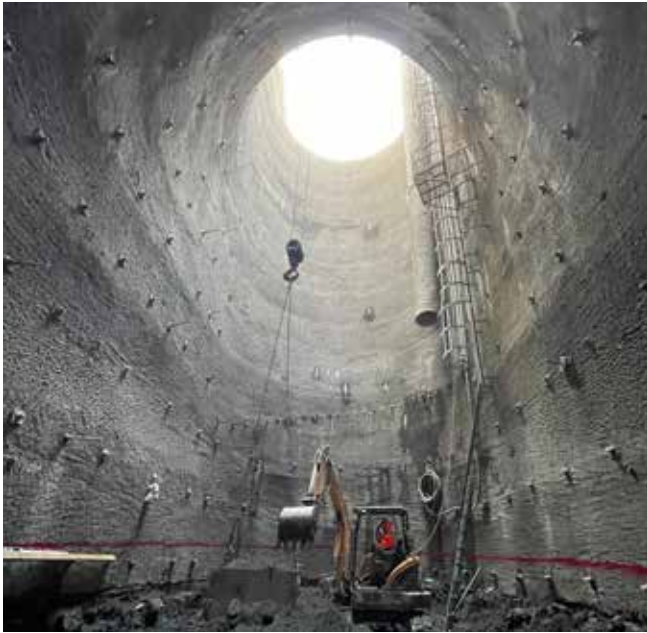
LEFT: Looking up into the 9 in. thick shotcrete lined 105 ft deep variable shaped shaft
