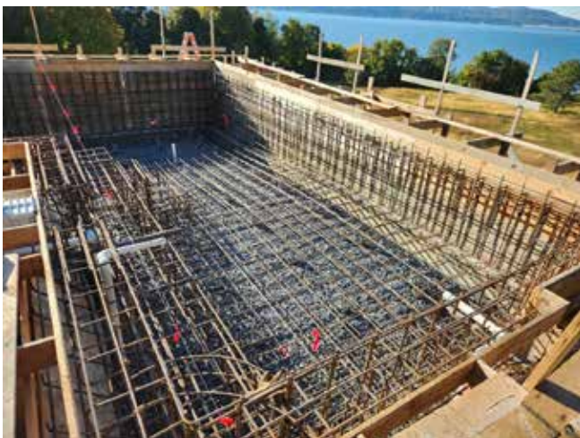
Fig. 5: Forming, plumbing out steel installation on top of cast foundation support for the wet-mix shotcrete methodology
