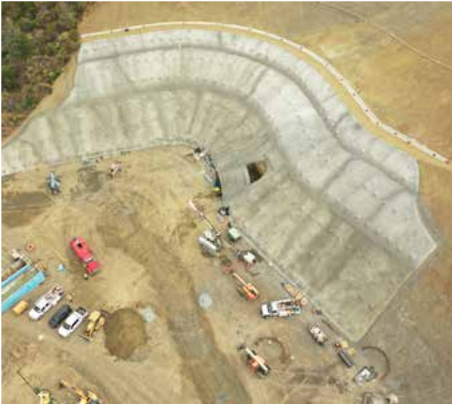
Aerial view of the 48,000 ft 2 (4500 m 2 ) soil nail & reinforced shotcrete portal and the beginning of tunnel excavation
