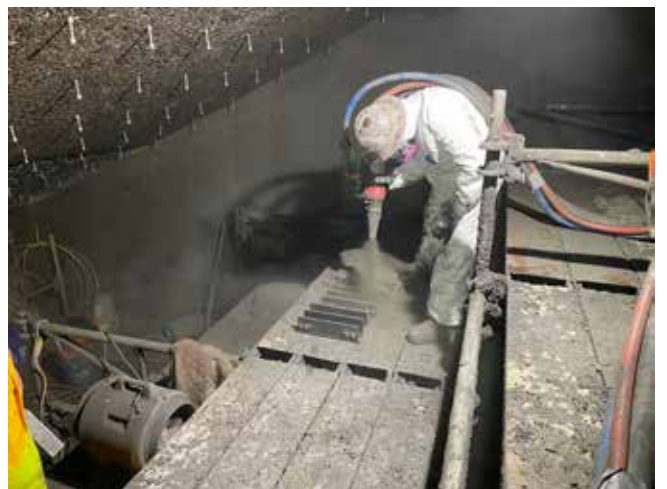
Beam molds shot for determination of early age compressive strength using end beam tester
