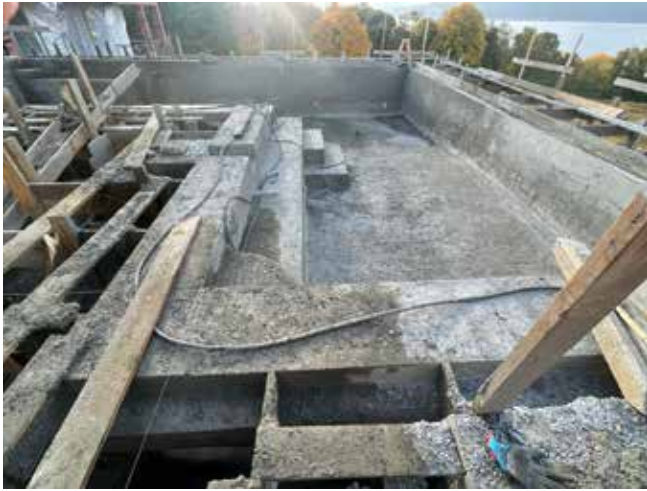
Fig. 6: Form removal, quality concrete example of the wet-mix shotcretes with soaker hoses for curing in place
