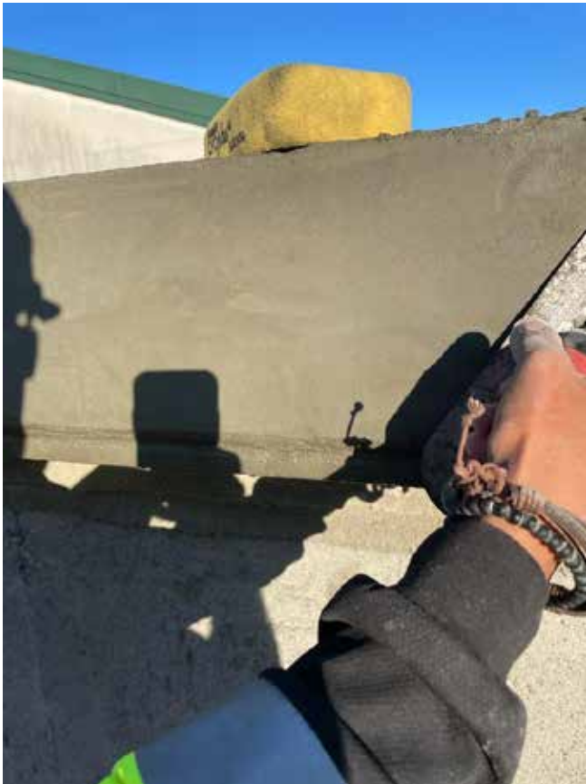
Fig. 6: Smooth steel trowel and sponge float used to finish concrete beams for a precast look and feel.
