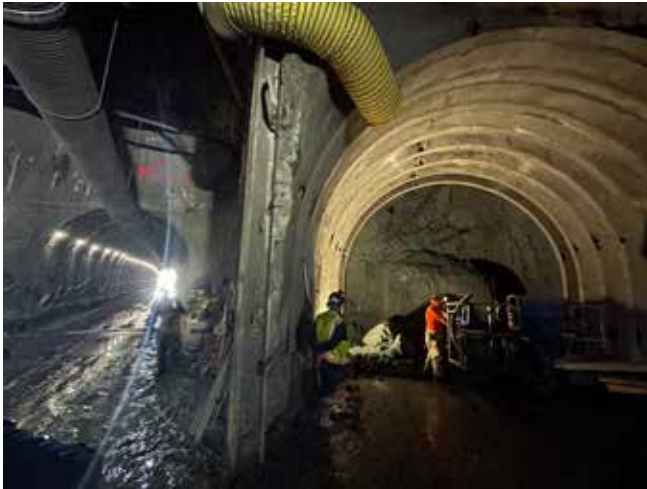
Photo taken viewing tunnel bifurcation/intersection area, shotcrete liner visible in both tunnels
