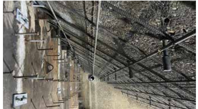
Permanent steel form, one-inch diameter anchors, and #5 reinforcing steel mat installed, secure and ready for shotcrete
