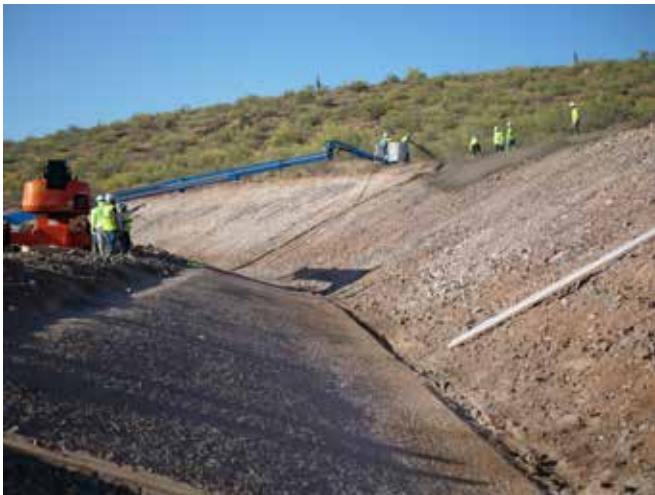
V-Ditch Shotcrete Installation: BAM Shotcrete crew installing a durable shotcrete lining in a V-ditch for enhanced water flow management and erosion resistance.
