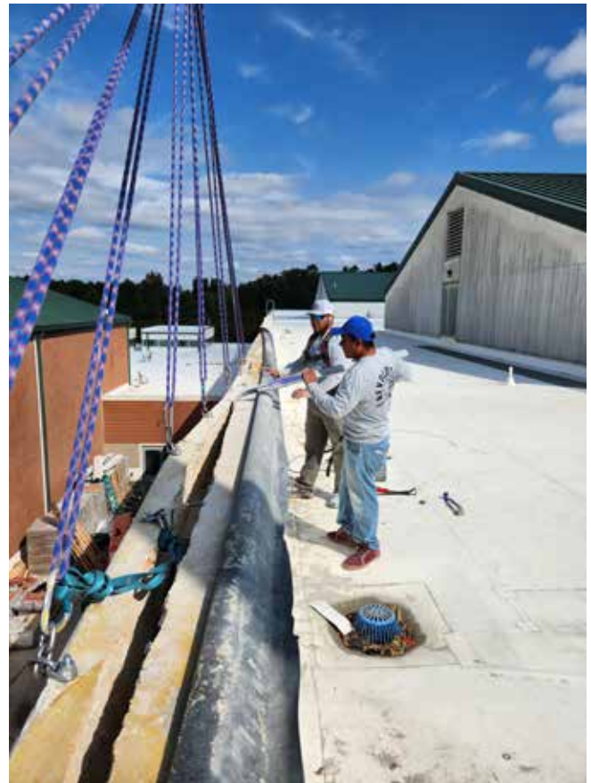
Fig. 7: Removing the decorative concrete beams, with equalized anchor points, by crane. Once under tension, the workers could pry the cracked beam off the safety bolts. The beams were then lowered into a dumpster with minimal effort. No pieces were dropped to the ground below.
