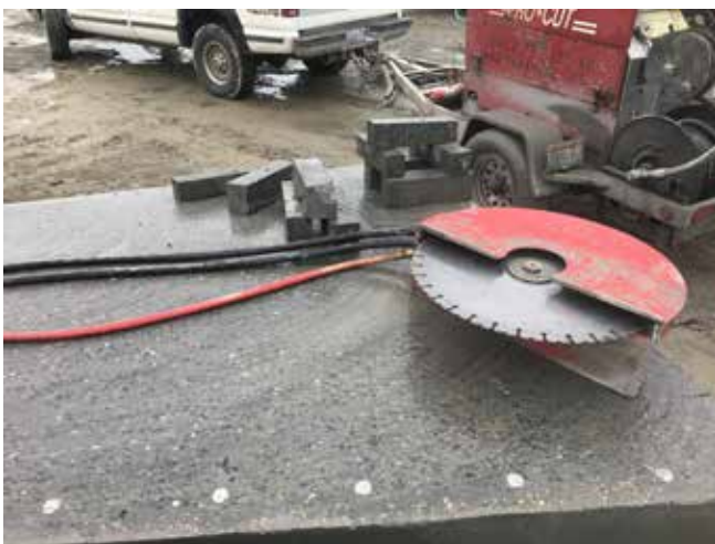
A diamond wire cut section of a full-scale mock-up showing excellent shotcrete consolidation around rebar and saw cut prisms for bond testing
