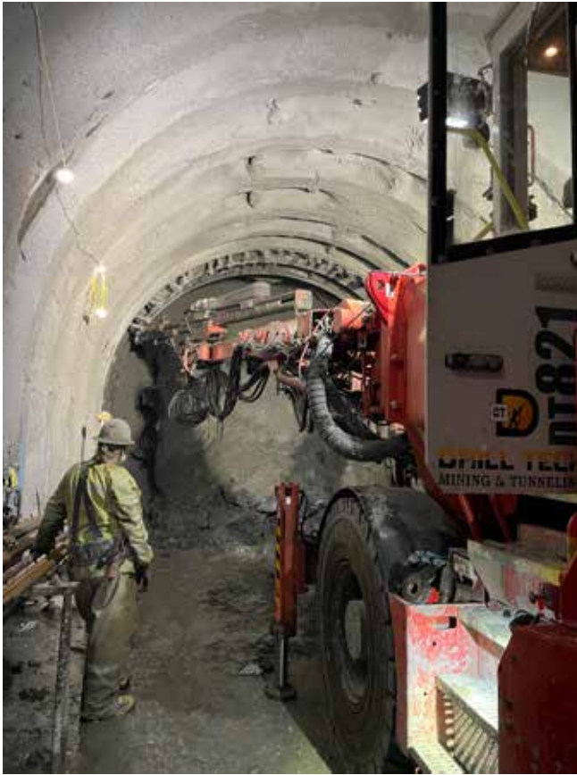
Two-boom jumbo installing pre-support spiles over steel set arches and shotcrete tunnel lining
