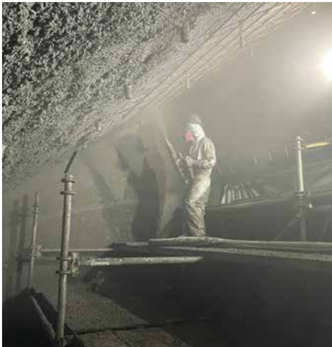
Shotcreter shooting overhead on a scaffold platform in an upright position to the No. 5 rebar and the one-inch anchors
