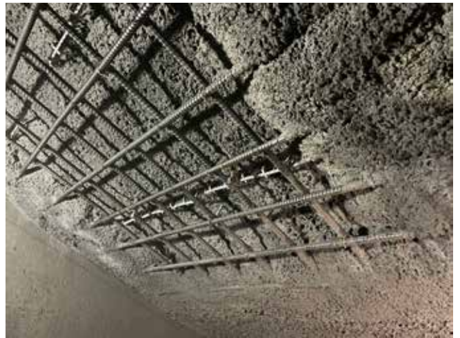
Excellent quality of encasement of the No. 9 rebar was observed by the shotcrete inspector
