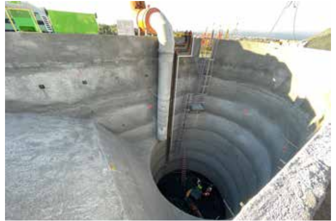
BELOW: Looking down into the 9 in. (230 mm) thick shotcrete lined 105 ft (32 m) deep variable shaped shaft
