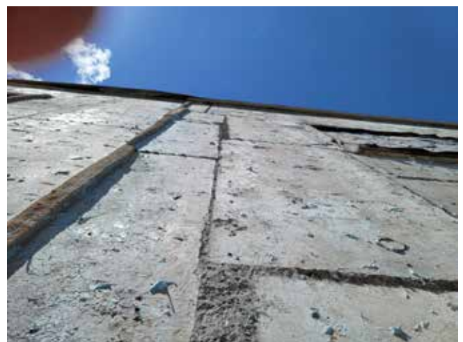
Fig. 5: Wavy foam molded tilt-up concrete substrate, undulating up to 2.5 in. in any direction.
