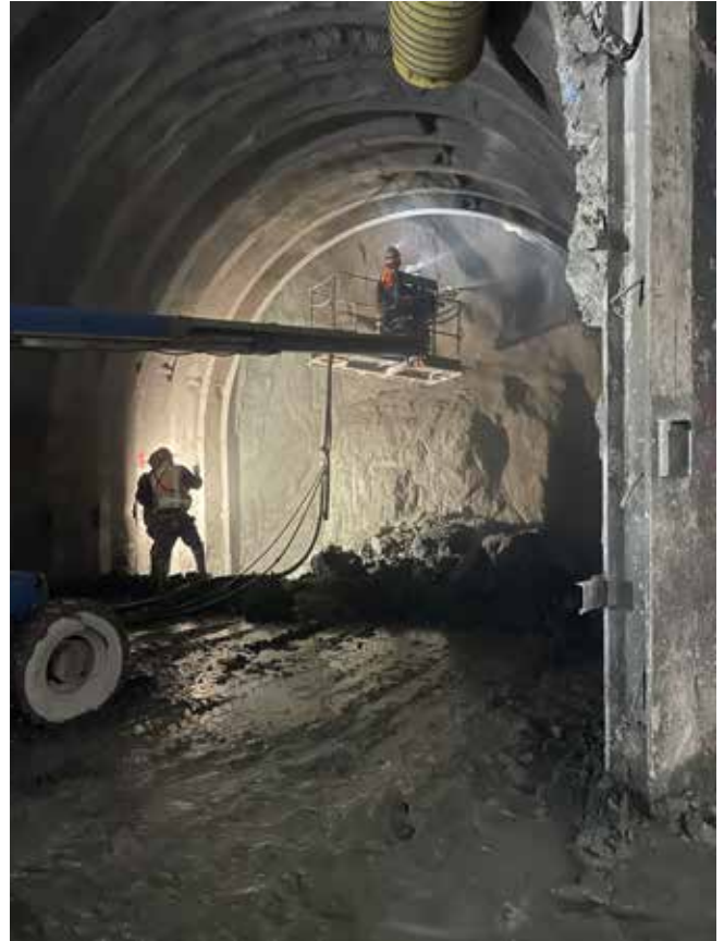
Tunnel Shotcrete placement via manlift and hand nozzle in 24 ft diameter tunnel
