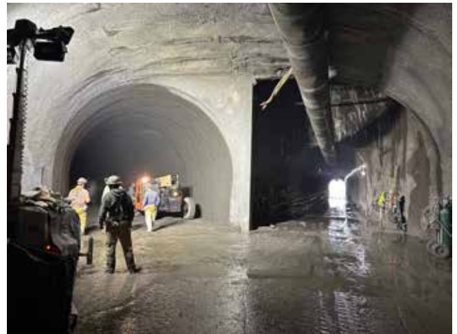
Looking into the Transition Zone bifurcation/intersection; comparison of complete smoothing shotcrete on left side and the in-progress right side which had yet to be completed
