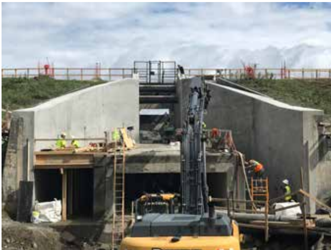
Downstream dam elevation revealing the culvert below and the training wall detail
