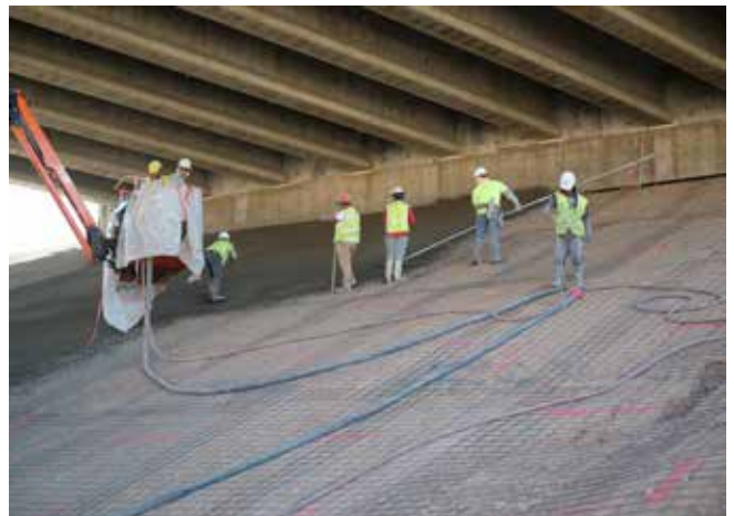
Bridge Scour Protection: Skilled BAM Shotcrete crew applying shotcrete to protect the bridge foundation from erosion and water damage, securing long-term stability.
