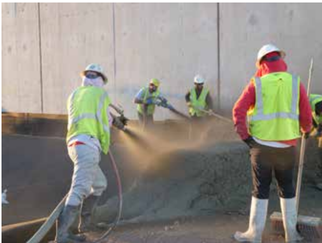
Shotcrete Oil Pit Installation for Transformer Switchgear: Workers installing a robust oil containment pit using shotcrete, designed for safety and environmental protection in industrial applications.
