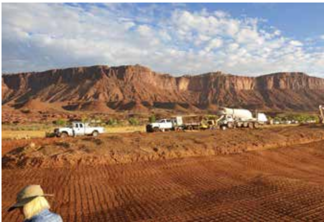
Artificial River Constructed for Kevin Costner's Movie: A scenic artificial riverbed, crafted using concrete and shotcrete techniques, set against the Utah landscape for the Netflix movie, Horizon: An American Saga .
