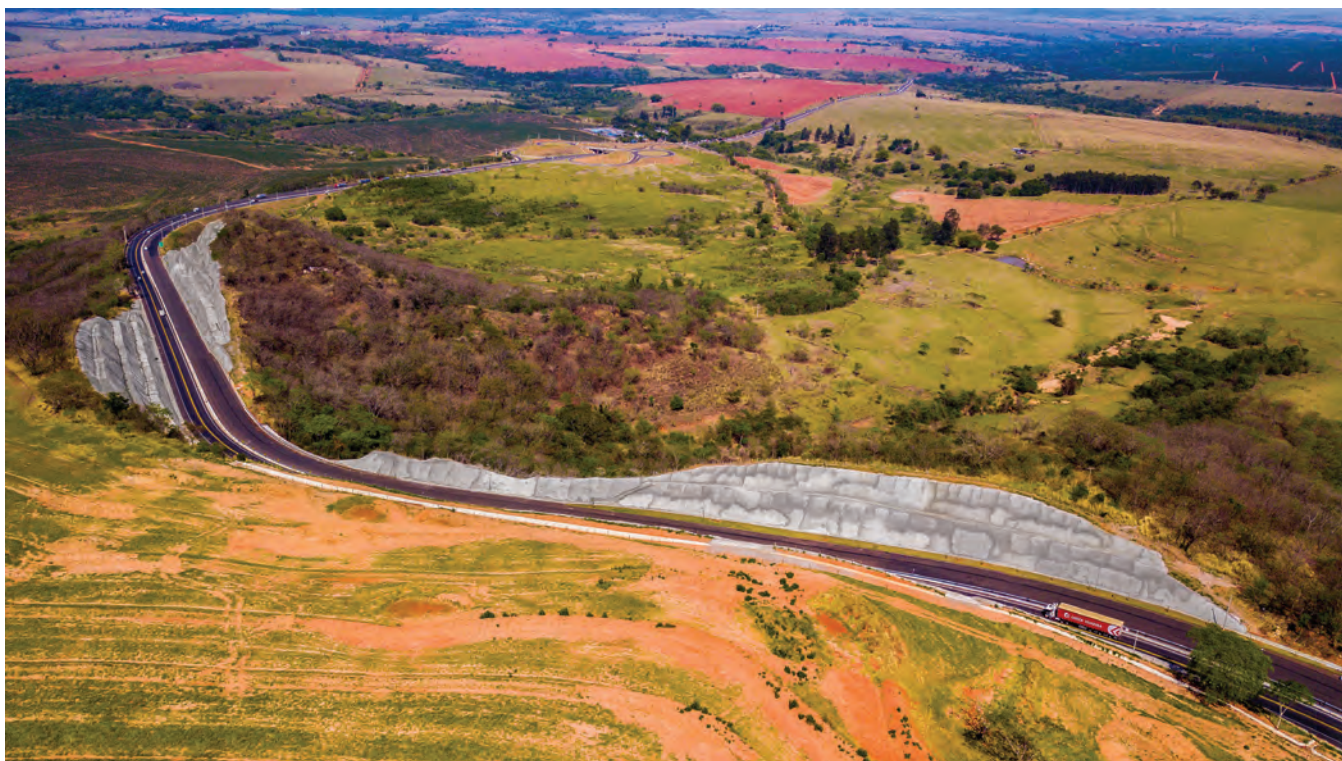
Fig. 1: Completed roadside slope connecting the towns of Marília and Assis in the state of São Paulo, Brazil.
