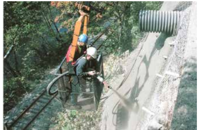
Slope stabilization in Westernport, MD. One of the advantages of shotcrete is being able to effectively place material in hard to access areas.
