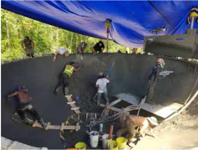
A Bowl-in-One! Kaaterskill Kahcrete and Nor'easter Skateparks shape artist Chemi Rosado-Seijo's "The Ceremonial Bowl" at Art Omi in Ghent, NY. Photo credit: Bart Friedman
