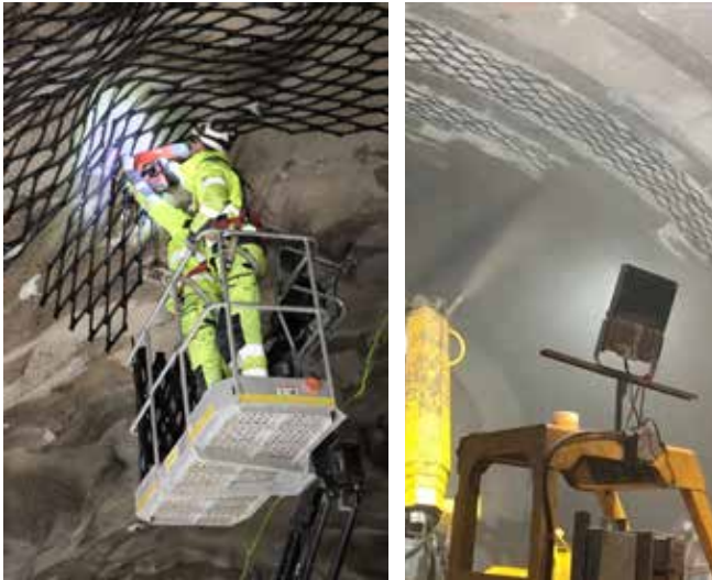
Fig. 5: Installing Dolenco Drain to tunnel crown and next covering with another layer of shotcrete.
