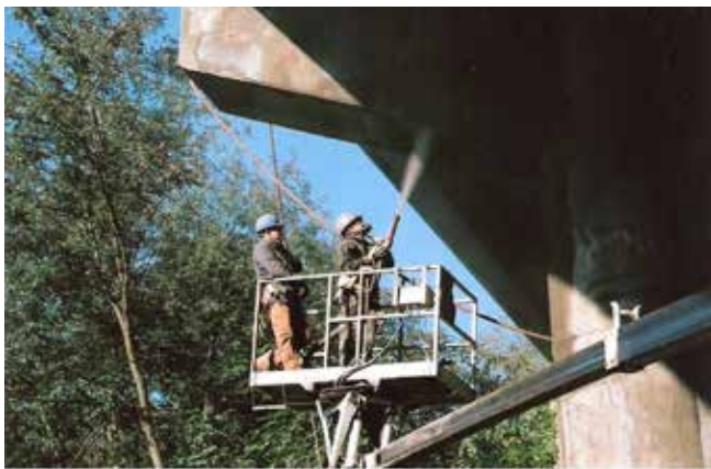
We needed to educate people about the advantages of shotcrete, such as the ability to place material overhead, as on this bridge hammerhead outside of Pittsburgh, PA.
