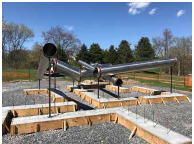
Mirror finished stainless steel pipes from Poland, suspended in place before shotcrete application.
