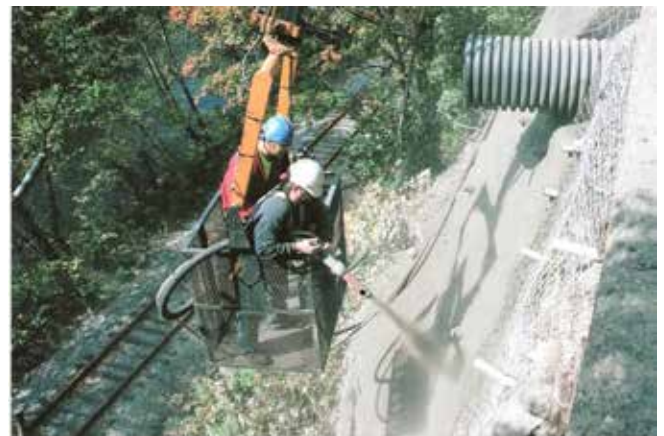
Slope stabilization in Westernport, MD. One of the advantages of shotcrete is being able to effectively place material in hard to access areas.
