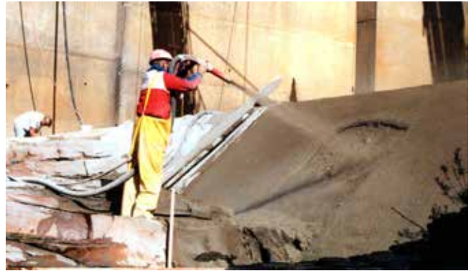
Dry Process Shotcrete repairs on the base of a dam in central Pennsylvania. Conveying and efficiently placing material is one of many hidden advantages of using shotcrete.
