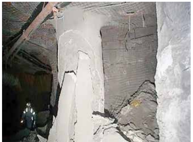
Fig. 5: Pillar collapse due to the lack of reinforcing steel
