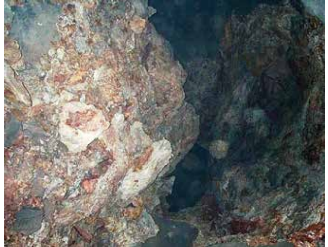
Fig. 4: Very-thin shotcrete caused a mine collapse
