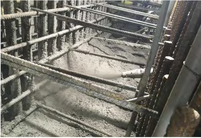
Fig. 19: Inspectors inside the wall observing nozzleman inserting the nozzle with the pipe extension through the opening in the front mat of steel to reduce the shooting distance to the back of the work.
