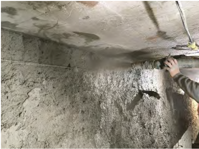
Fig. 10b: Shooting to the StayForm and out to cover the front reinforcing steel and up to the roof.
