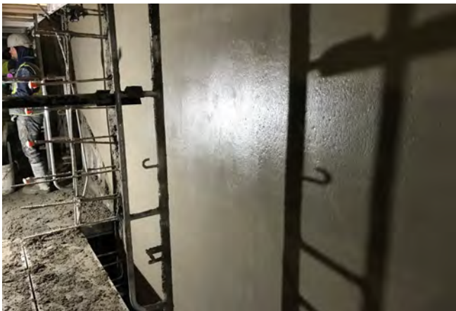
Fig. 16: Final finished surface at the West Headwall tunnel openings. Credit: Jimmy Wang.
