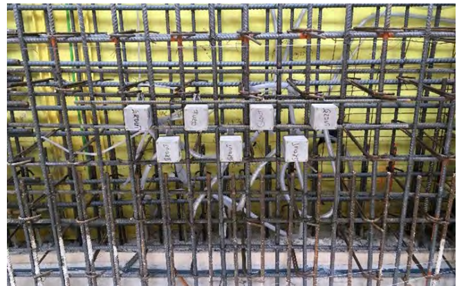
Fig. 11b: Waterproofing system consisted of a post curtain wall grouting capability and many grout tubes and injection boxes fastened to the reinforcing steel.
