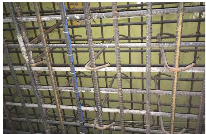
Fig. 12: A BA Anchor (red arrow) and rod spliced to a hook bar is shown and was used to brace the wall to resist forward toppling.
