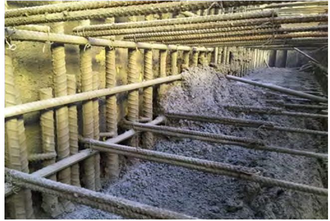
Fig. 20: Inspectors inside the wall observing operator inserting a long stiff rod vibrator right to the back of the work to provide the shotcrete in place with supplementary consolidation.
