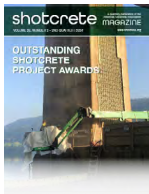
2023 Honorable Mention Project, the Neville Island Bridge | Coraopolis, PA: Installing Shotcrete from a barge in the main channel of the Ohio River.
