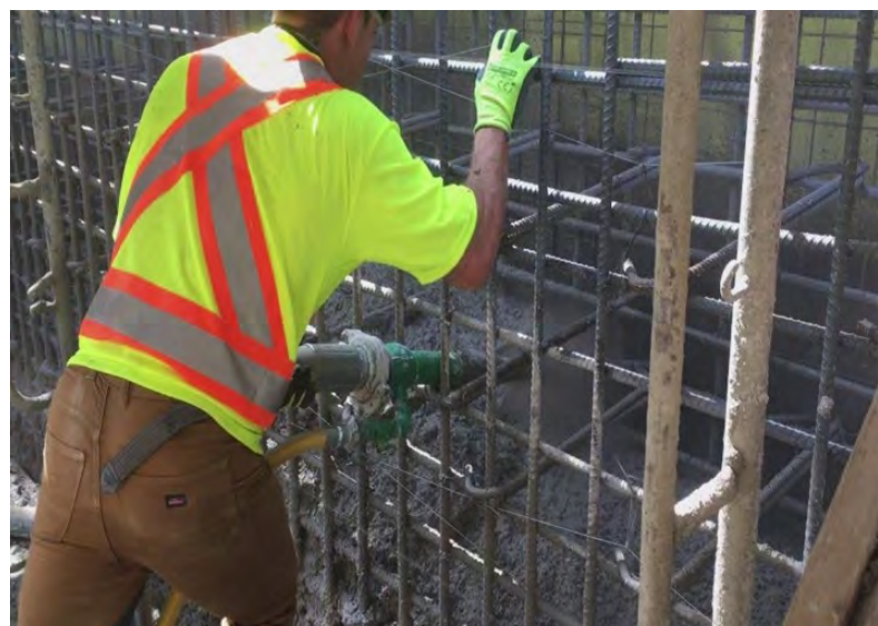
Fig. 18: Inspectors would be up close and provided with a “birds eye” view of shotcrete being applied by the prequalified ACI-certified nozzleman. Shotcreter bench shooting to the back of the work.
