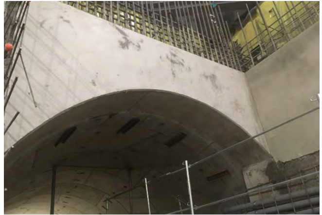
Fig. 23: Mount Pleasant Station, and a close-up view of the tunnel arch that was constructed using the “hybrid” shoot and then vibrate shotcrete process for the West headwall.
