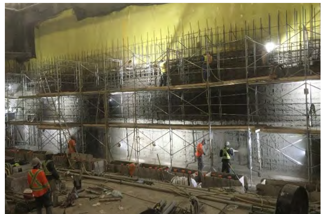
Fig. 9: Large shotcrete volumes of up to 224 m 3 were applied in a single day of production at Mt Pleasant Station in Toronto using two pumps and shotcrete crews.
