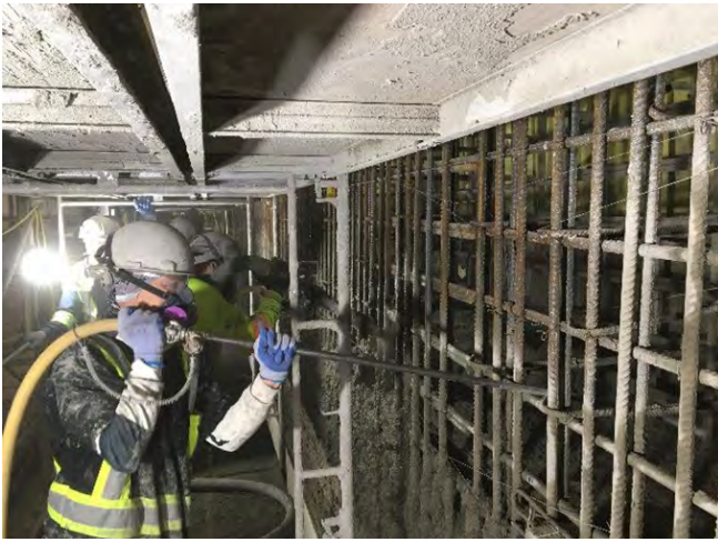
Fig. 6: Compressed air blow pipe working in tandem with shotcreter during bench shooting.
