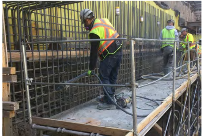
Fig. 15: Shotcreter bench shooting (background) followed by an operator with a long stiff rod vibrator (foreground) being inserted into the work to provide the shotcrete with supplementary consolidation around the back reinforcing steel.
