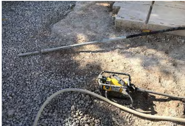
Fig. 7: A long 40 mm (1.6 in.) diameter stiff rod vibrator for supplemental consolidation. Credit: Jimmy Wang.
