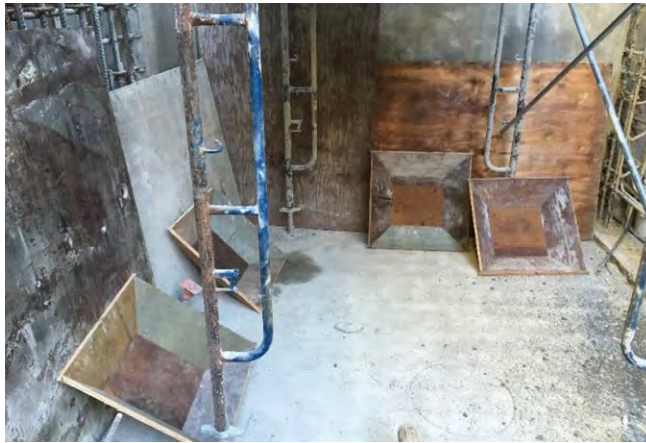
Fig. 21: Production test panels ready to be shot for taking cores and evaluating compressive strength of the concrete material at 7, 14, 28 and 56 days.
