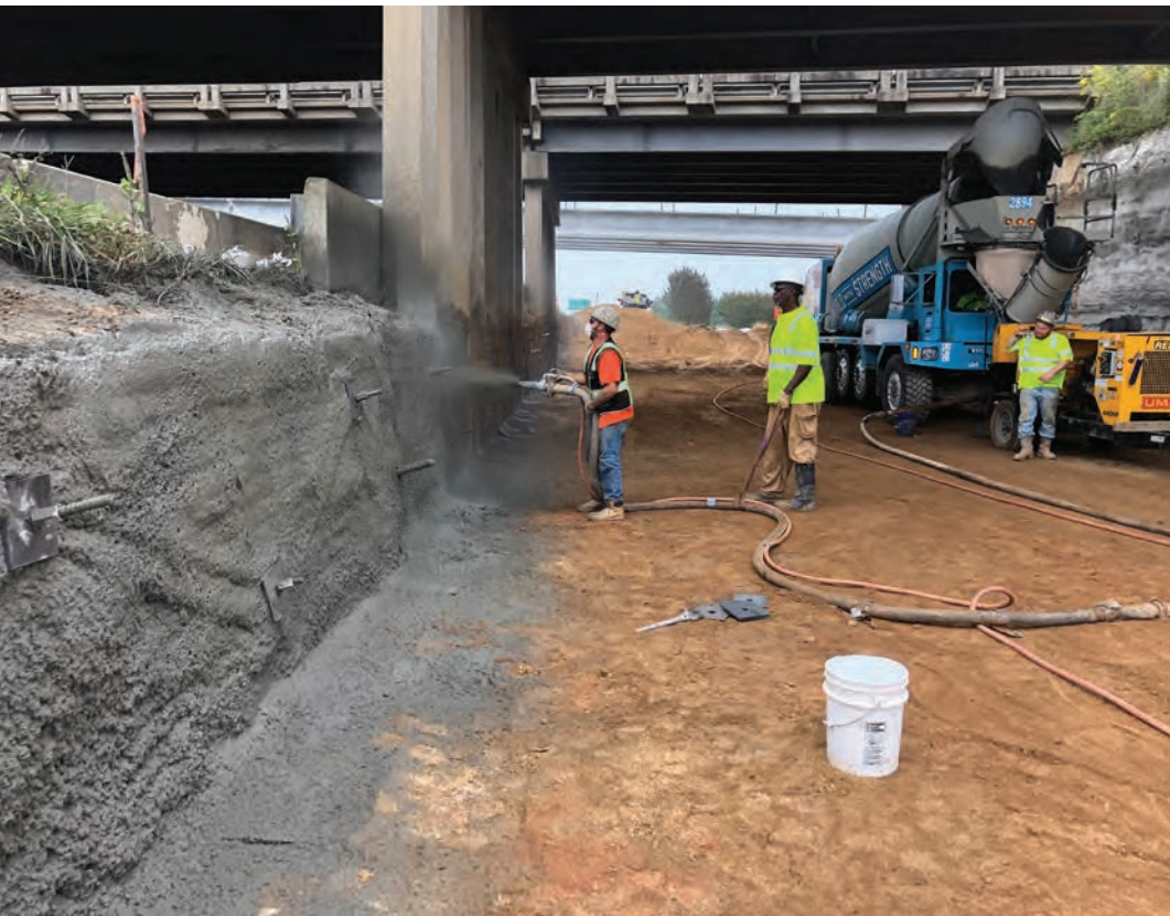
UMA's earth retention and sculpted shotcrete work on NCDOT's I-40/I-77 interchange improvements project held up cuts for widened roadway sections and facilitated new bridge construction.
