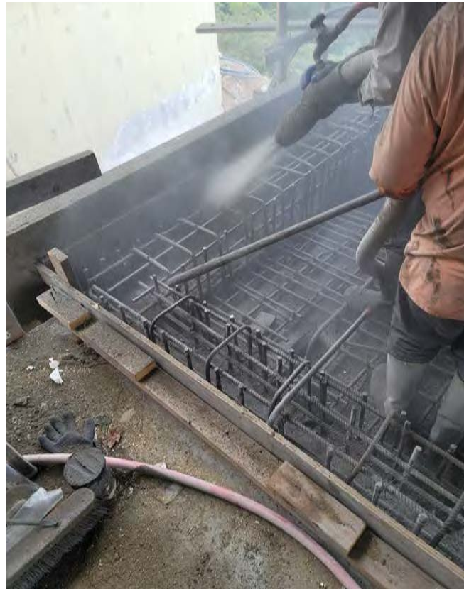
Fig. 4: Air lance operator keeping the corner free from rebound until the nozzle man places material in the corner. High quality diaphragm water valve ensures a sensitive control of mix water
