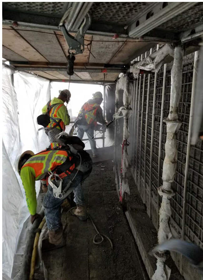
Fig. 10: Extensive containment measures taken to control overspray and protect surrounding structures during shotcrete application
