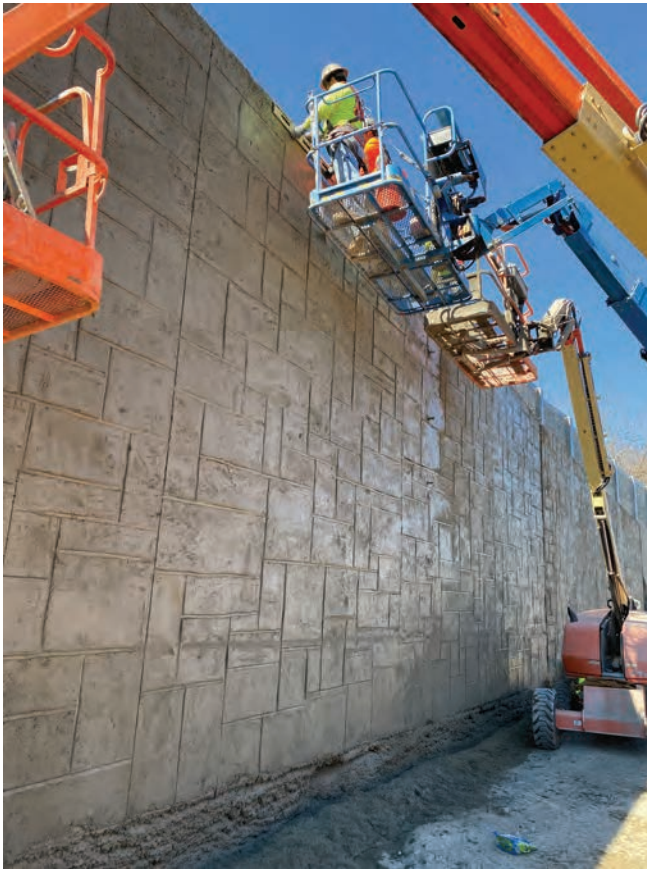
Craftspeople in man baskets performed all sculpted shotcrete work by hand, from spraying material to carving the artistic patterns.
