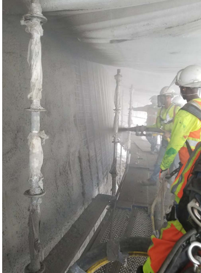
Fig. 9: Shotcrete application, note extensive containment to control overspray and protect surrounding structures
