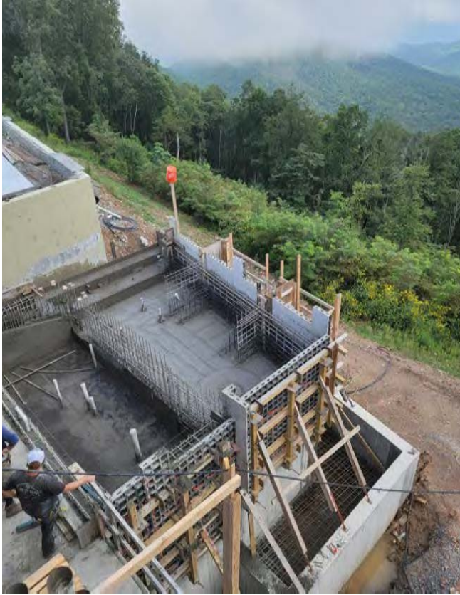
Fig. 2: First the pool floor was shot along with a gutter wall, which allowed the forming of the shelf and additional bar
