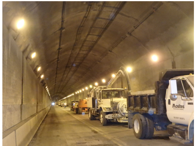
Fig. 3b: Ceiling removed in Eastbound - The concrete in the older, eastbound tunnel was not air-entrained so the cracking of the ceiling was far more extensive; here we see the tunnel with its ceiling removed.
