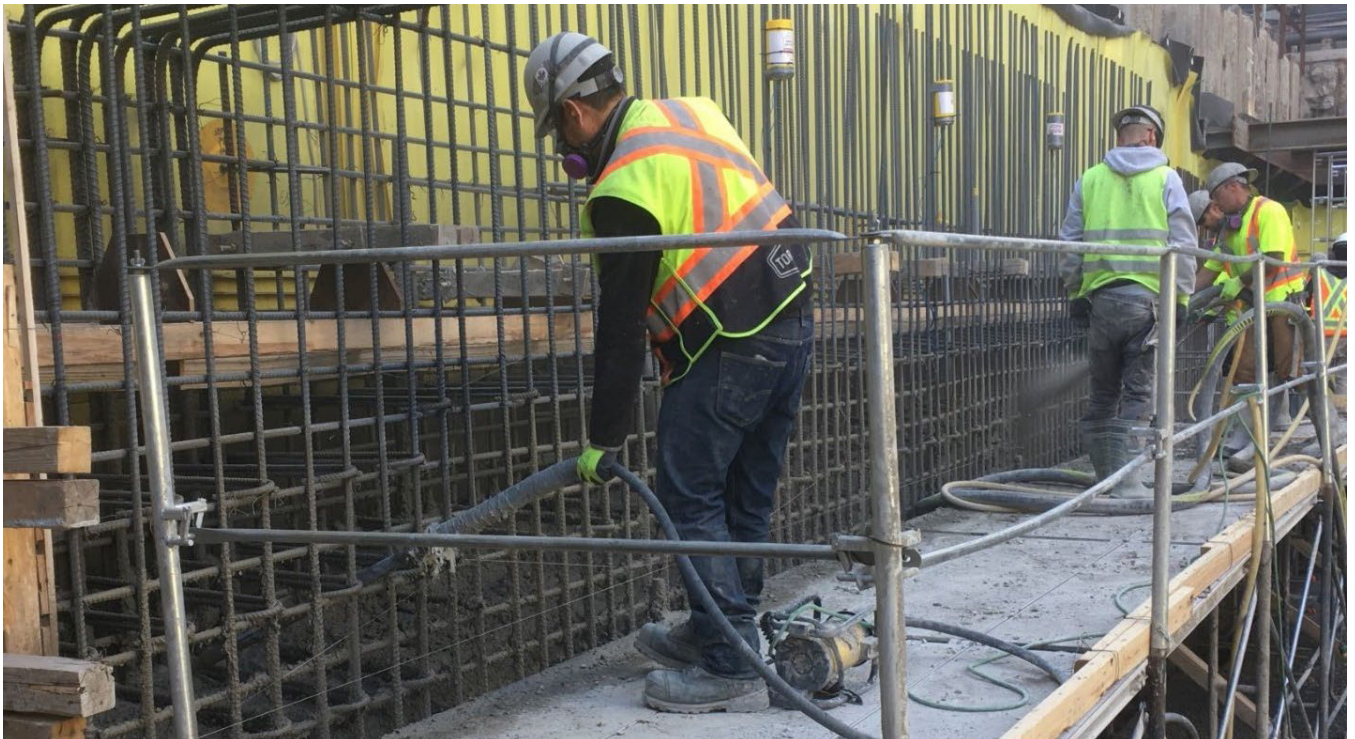
Fig. 10: A close-up view of the shotcrete contactor's nozzleman bench shooting (background) followed by an operator of a long stiff rod vibrator (foreground) being inserted into the work to "lay down the bench" and provide the shotcrete with supplementary consolidation around the back reinforcing steel.
