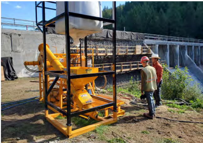
Fig. 7: Bulk bag hanger at Moyie Dam, 2021.
