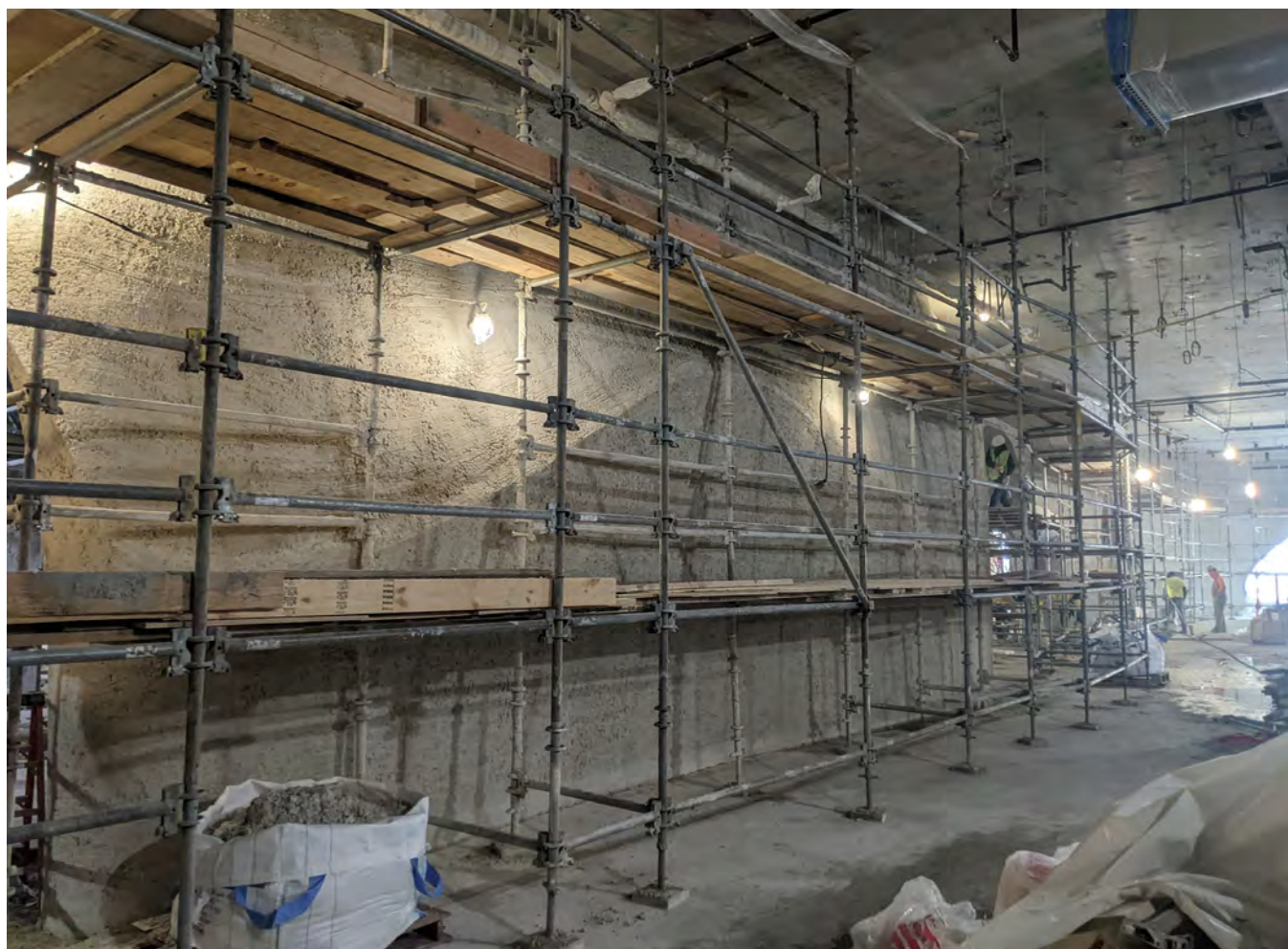
Fig. 8: After structural coat was set, shoring could be removed. This allowed for ample room to shoot the finish coat.
