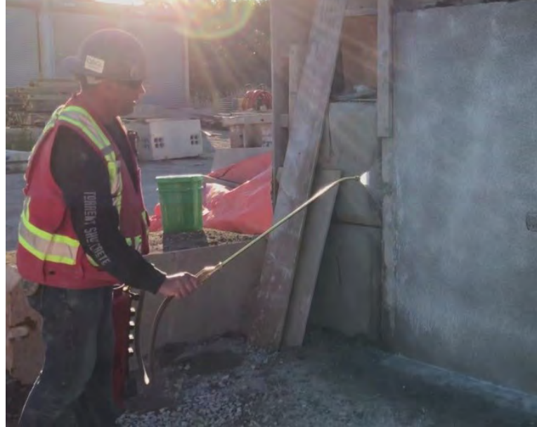
Fig. 18: Finished mock-up was cured using a spray on applied curing compound. Photo Credit: Jimmy Wang.
