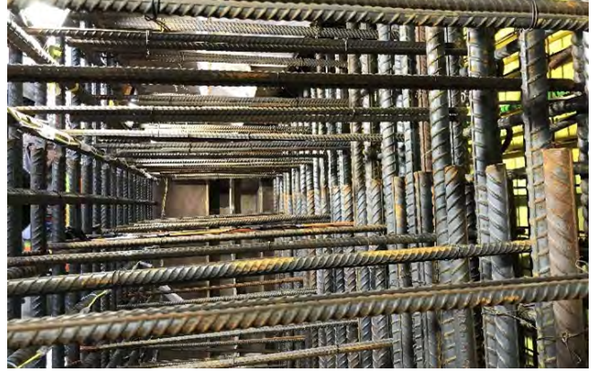
Fig. 9: Inside mock-up showing spliced 25M vertical reinforcing (inner wall face), spliced 3-35M vertical reinforcing (outer wall face), 15M holder bars and plastic waterstop.
