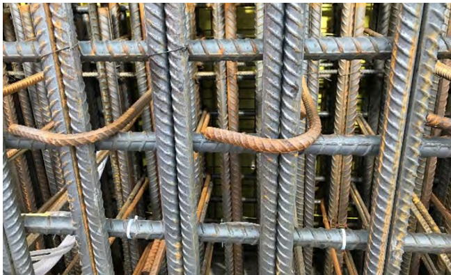
Fig. 8: Mock-up was heavily reinforced with 4 layers of heavy rebar, including 3 layers of closely spaced 35M (#9) rebar at the back of the work adjacent to a water proofing membrane. Photo Credit: Jimmy Wang
