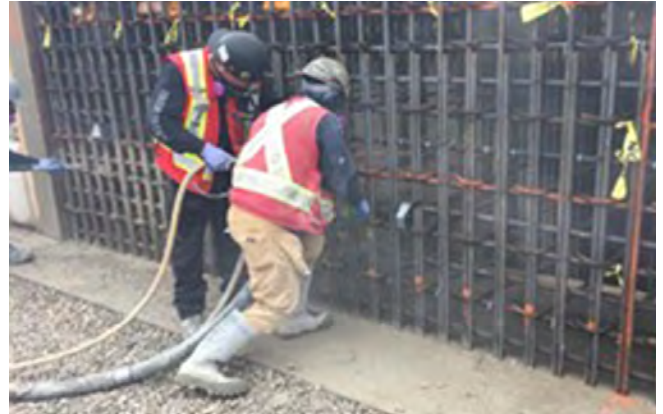
Fig. 10: Nozzleman bench shooting mock-up with blow pipe operator working in tandem with the nozzleman.
