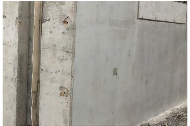
Fig. 19: Finished mock-up following stripping of the formwork after curing in air for 10-days.
