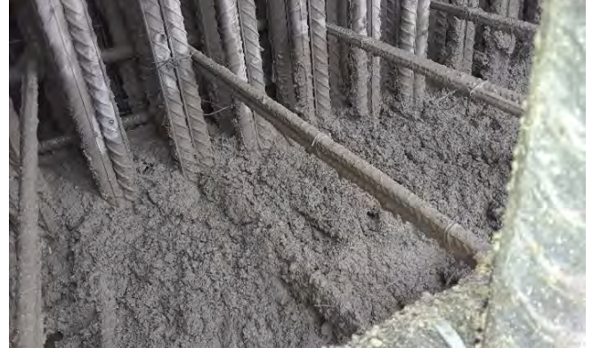
Fig. 14: Following use of stiff rod vibrator, shotcrete was being well consolidated and wrapping around the three outer 35M reinforcing steel bars. Photo Credit: Leonard Crasta.
