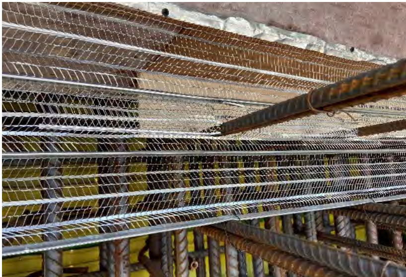
[Insert Figure 24] Fig. 24: A 300 mm wide StayForm positioned 450 mm. in from the front inner wall face used to act as a receiving surface to apply shotcrete out to cover the front rebar. Credit: Carl King.
