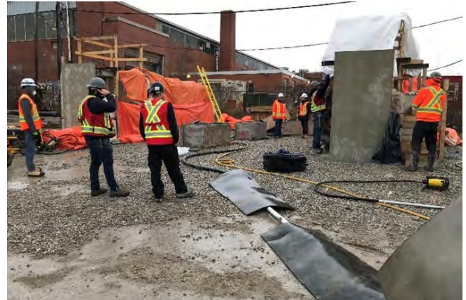
Fig. 4: Steel slickline and rubber hose which fed shotcrete to the mock-up. Credit: Jimmy Wang.
