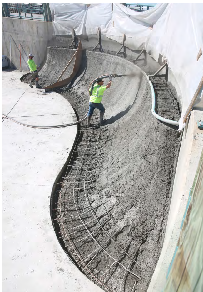
Fig. 7: Working the Wall—SR Crew Lead and ACI-certified Nozzleman Kelly Malobovich applies concrete to a crucial consolidation area beneath the steel coping of a new skate spot feature at the Redondo Beach Pier in California (2023). Project: Redondo Beach Pier Skatespot. Photographer: @Mikendo.
