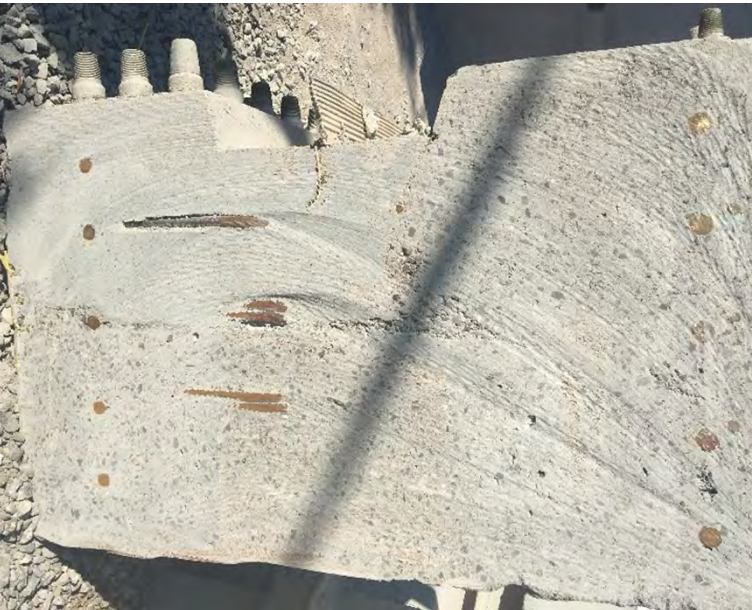
Fig. 23: An example of a wire saw cut section of mockup showing excellent quality of shotcrete at the transition between the shotcrete and the SCC using the StayForm Option 1 at the roof soffit with the keyway and plastic embedded water stop detail
