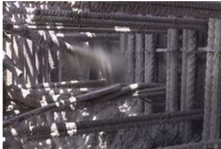
Fig. 11: Nozzleman inserting entire nozzle tip and extension between square openings in the front mat of reinforcing steel. Shotcrete stream impacting three layers of vertical reinforcing steel and water proofing membrane at a high impacting velocity. Blow pipe being used to continuously clean the back reinforcing steel in front of the area about to be shot.
