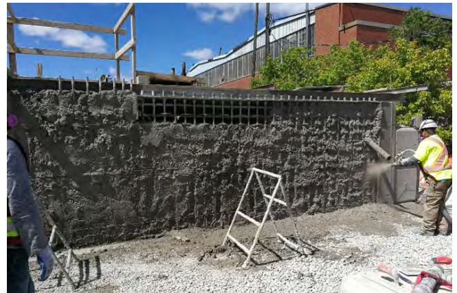
Fig. 15: Nozzleman shooting the final finish coat of the mock-up. Photo Credit: Jimmy Wang.
