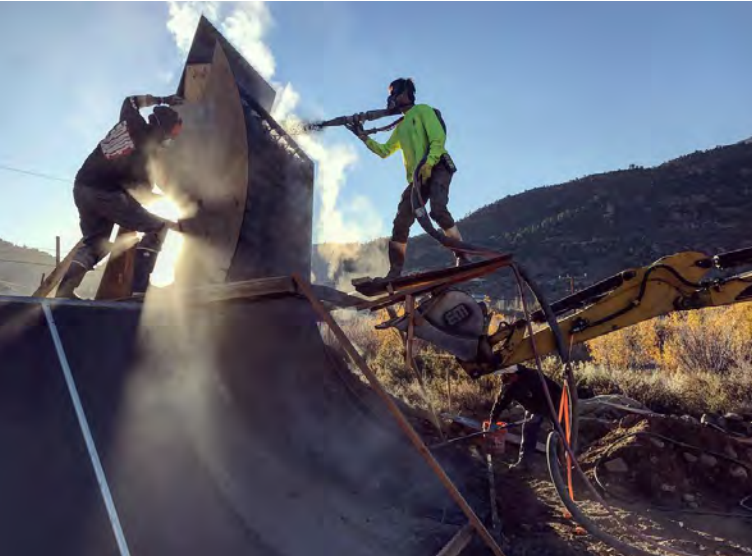
Fig. 9: Sunrise Silhouette—In the early morning light, Mark Bradford casts a shadow while he skillfully shoots a spray of concrete. Placement and consolidation are crucial. Project: Lake Crowley Skatepark, Lake Crowley, CA.
