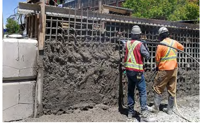
Fig. 13: Supplementary consolidation provided by insertion of a long 40 mm diameter stiff rod vibrator into the back of the work. Photo Credit: Robert Mattes.
