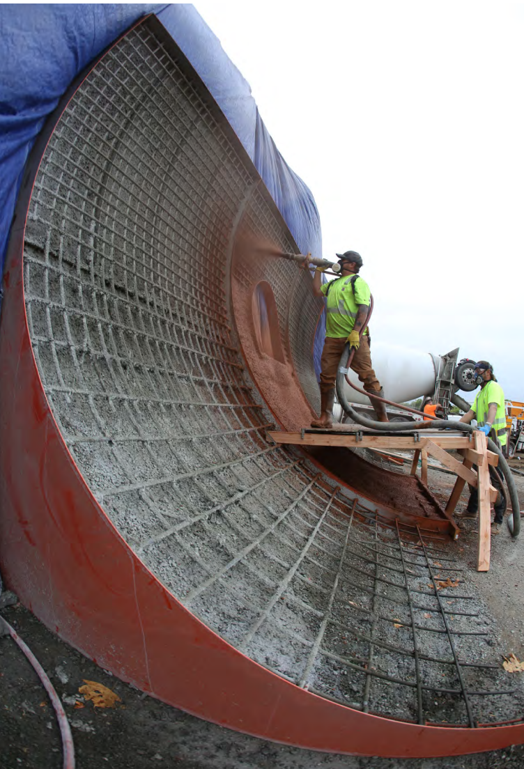
Fig. 3: A Cresting Vert Wall—SR Crew Lead and ACI-certified Nozzleman, Kelly Malobovich, sprays colored shotcrete onto an over-vert, free-standing concrete wall in La Puente, CA (2020). Project: Central Park Skatepark. Photographer: @Mikendo.
