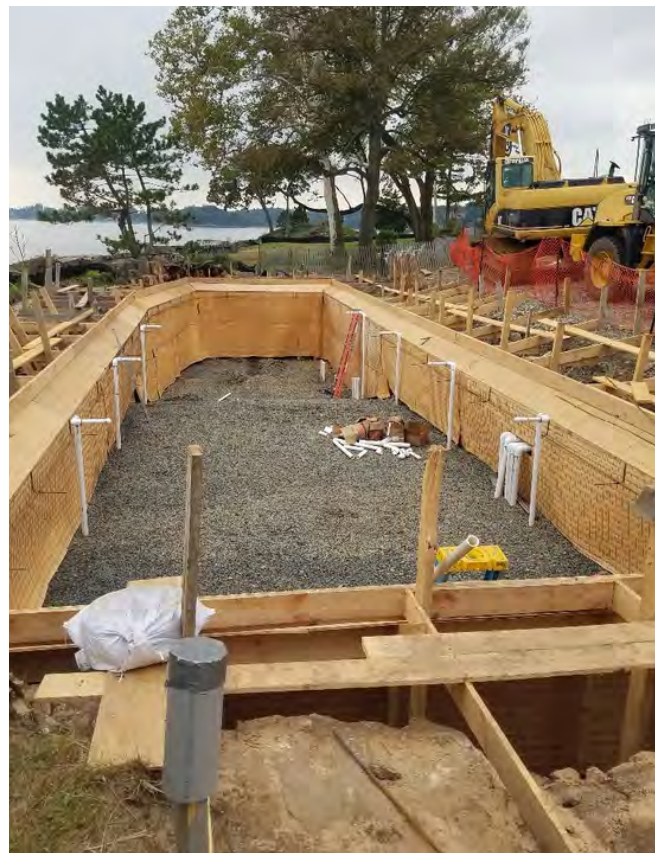
Fig. 6: So often, the true art and craft of construction resides in details that will go unseen once complete. The near-perfect formwork on this project is a prime example.
