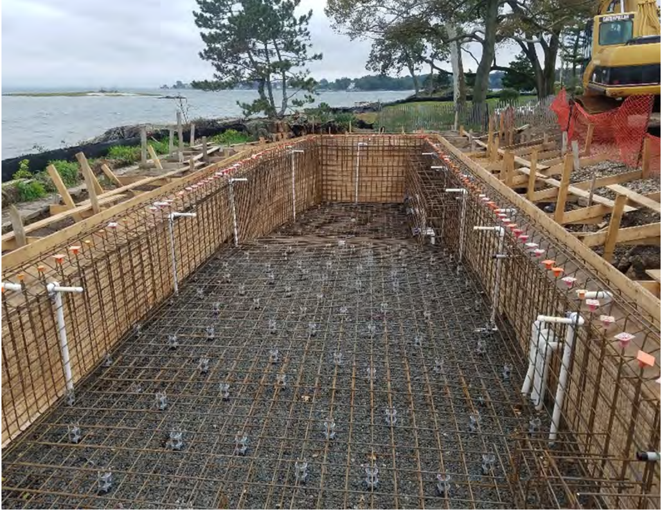
Fig. 7: It's a basic consideration, but properly elevating the steel above the ground is critical for structural integrity. Simple details matter. As is true of all-perimeter overflow systems, the forming, reinforcing steel, and shotcrete had to be installed to the highest possible standards and low tolerances. Suffice it say, this was not a job for a novice builder.
