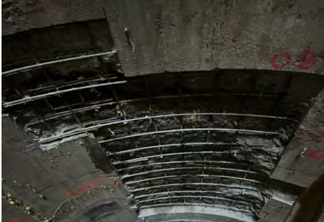
Fig. 5: Large repair that was converted from a form-and-pour to a shotcrete method repair.
