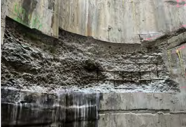
Fig. 4: Large Repair area.
