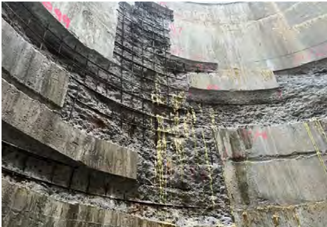
Fig. 3: Photo showing large repair areas with complex shapes making it difficult to form.
