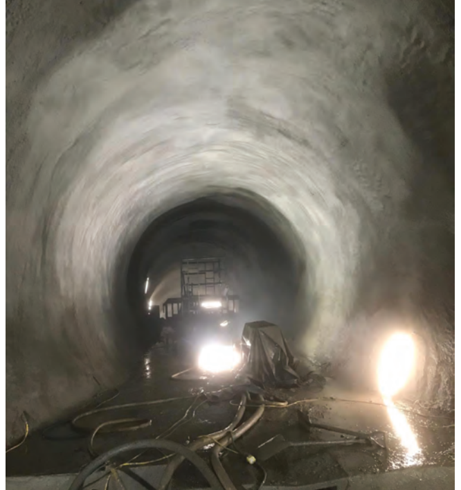
Fig. 7: Tunnel with lift and equipment
