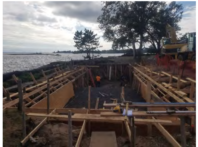
Fig. 5: That was not the situation here. The solid-rock shoreline in this area served as the form for the pool structure, an advantage that simplified the process.
