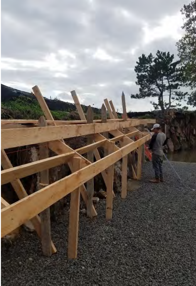
Fig. 4: Working so close to the shore can create challenges when it comes to the needed substructure and dealing with ground water or sandy soil conditions.
