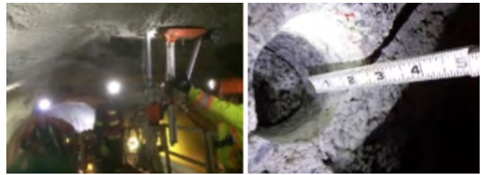
Fig. 9: In-place overhead shotcrete core extraction; visual inspection of core hole to evaluate shotcrete consolidation, shotcrete thickness, and bond.
