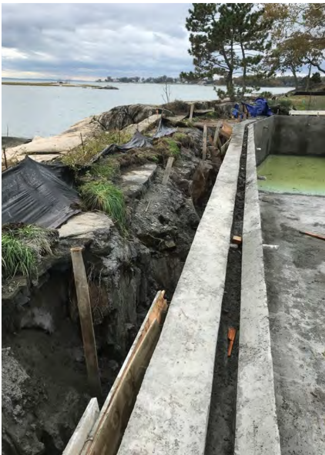
Fig. 3: Executing the precise edge detail required zero tolerance construction and dogged adherence to all applicable workmanship standards.
