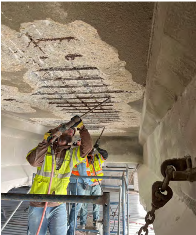
Figure 5: 2023, Chipping at Banks Channel Bridge, Wrightsville Beach, NC
