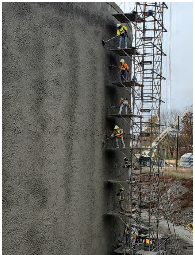
Figure 8: Scaffolding and finishers on a water tank; framed using the Rule of Thirds.
