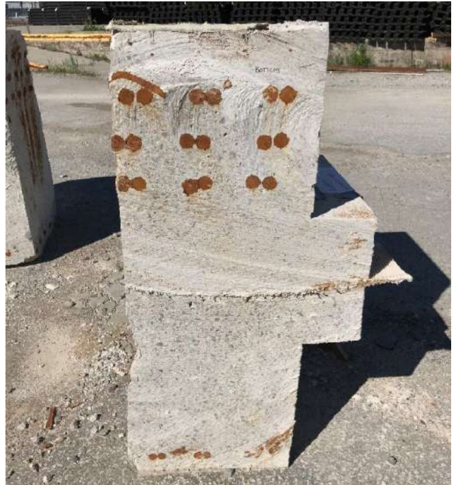
Fig. 8: A wire saw cut section of mockup showing excellent consolidation of shotcrete around the three layers of #35M (#11) rebar at the back of the work and to the outer membrane next to the embedded plastic water stop. Credit: Jimmy Wang.
