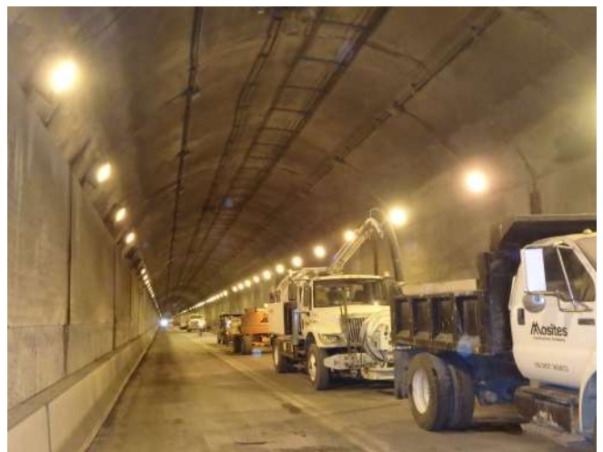
Fig. 3b: Ceiling removed in Eastbound - The concrete in the older, eastbound tunnel was not air-entrained so the cracking of the ceiling was far more extensive; here we see the tunnel with its ceiling removed.
