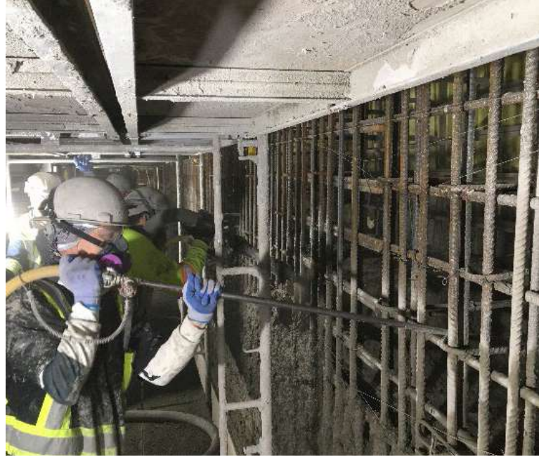
Fig. 4: Compressed air blow pipe working in tandem with nozzleman during bench shooting.
