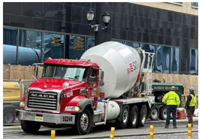
Fig. 4: Concrete being pumped down from the street plus 100 ft to the work zone.
