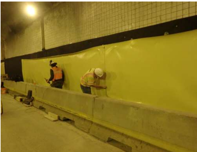
Fig. 5: PVC membrane installation - Specialist contractor Schneider-Moran is installing the first sections of waterproofing in the eastbound tunnel on the lower sections of tunnel wall.
