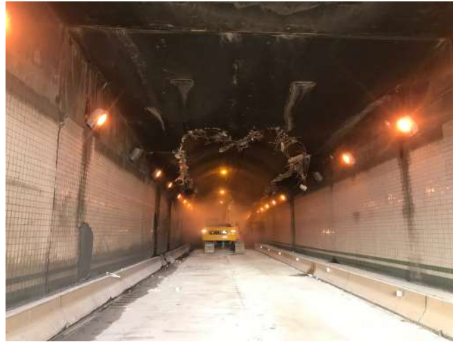
Fig. 3a: Work underway in Eastbound - Mosites has removed the ceiling and the barriers at either side of the tunnel. Each weekend, the tunnel must be reopened to traffic.
