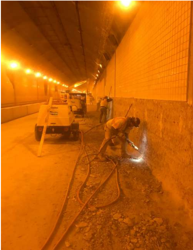
Fig. 4: Demolition 1 - The barriers at the side of the eastbound tunnel were removed so that the new waterproofing system could be installed.
