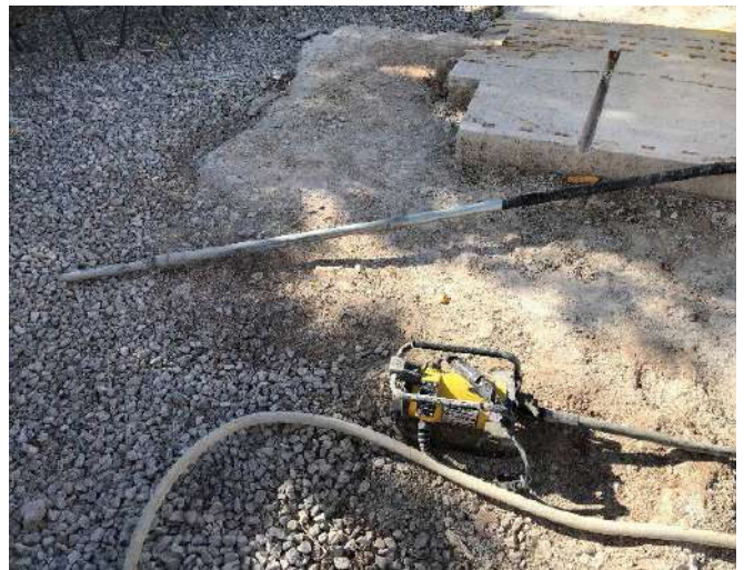
Fig. 5: A long 40 mm (1.5 in.) diameter stiff rod vibrator provided the placed shotcrete with supplementary consolidation. Credit: Jimmy Wang.
