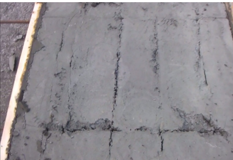
Fig. 6b. Further evidence of tracking visible from the formed side.
