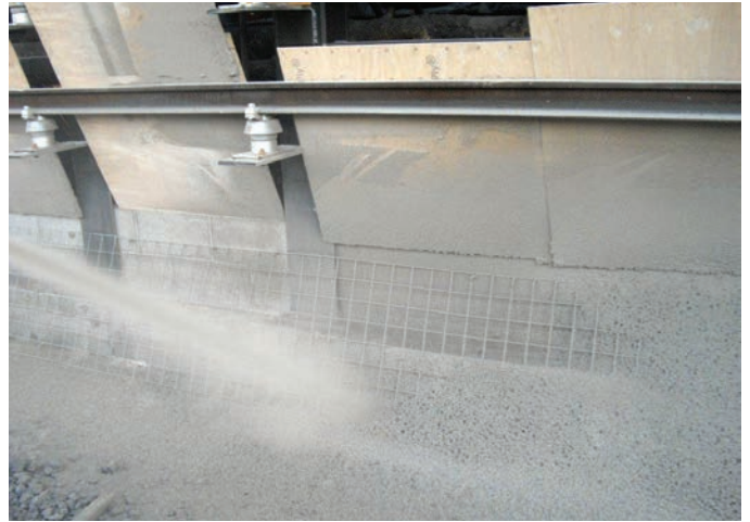
Shotcrete is gunned at high velocity onto the receiving surface. On initial impact, a larger percentage of aggregate rebounds from the surface, leaving a thin layer of cement paste at the interface of the new shotcrete and the substrate
