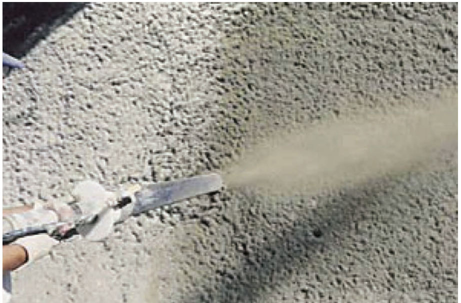
High-volume wet-mix shotcrete with large aggregate is evident in the texture of the material already placed
