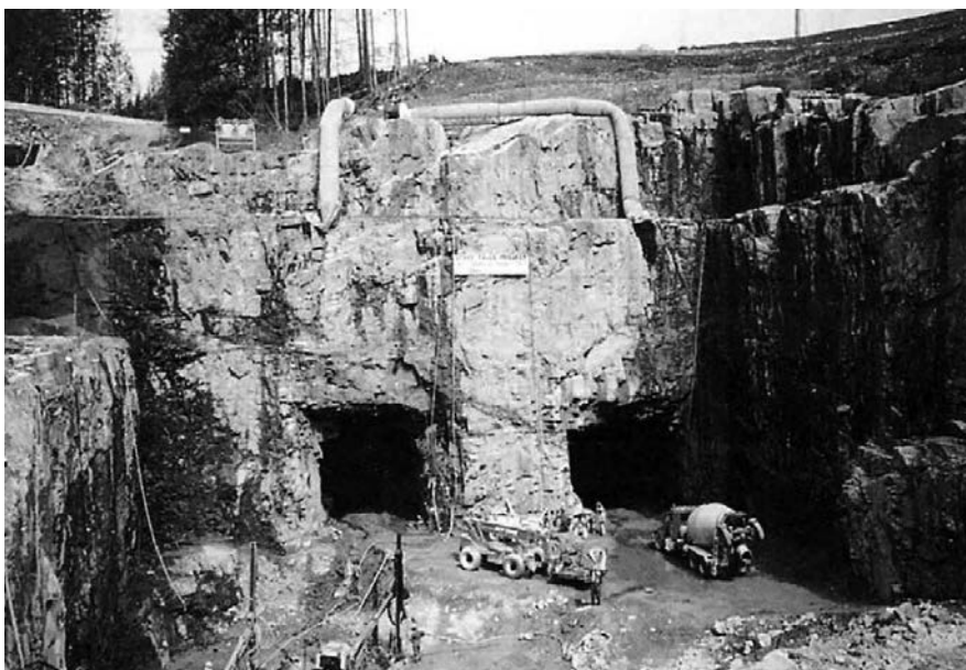
BC Hydro Stave Falls Hydroelectric Project: Downstream outlet of SFRS-lined pressure head race tunnel.
