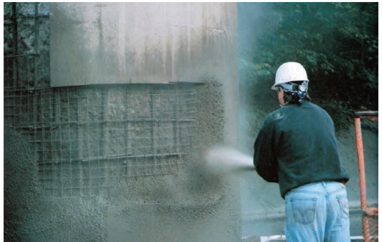
The dry process of shotcrete being gunned on a pier can provide a better bond without using bonding compounds. The nozzle man is filling in the corners first and working toward the middle of the repair area so he doesn't trap rebound in the corners
