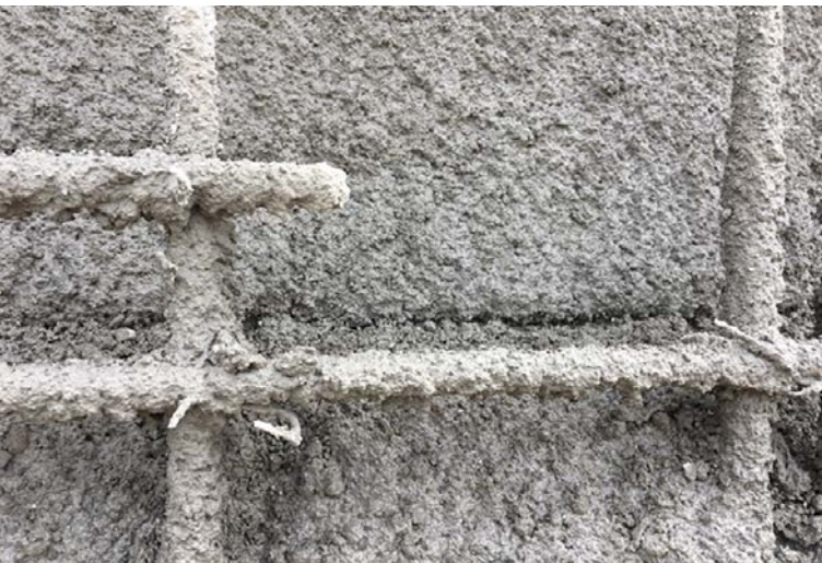
Fig. 6a. Tracking occurring within the shadow area is easy to see. Tracking behind reinforcements is visual evidence that the mixture is far too stiff.
