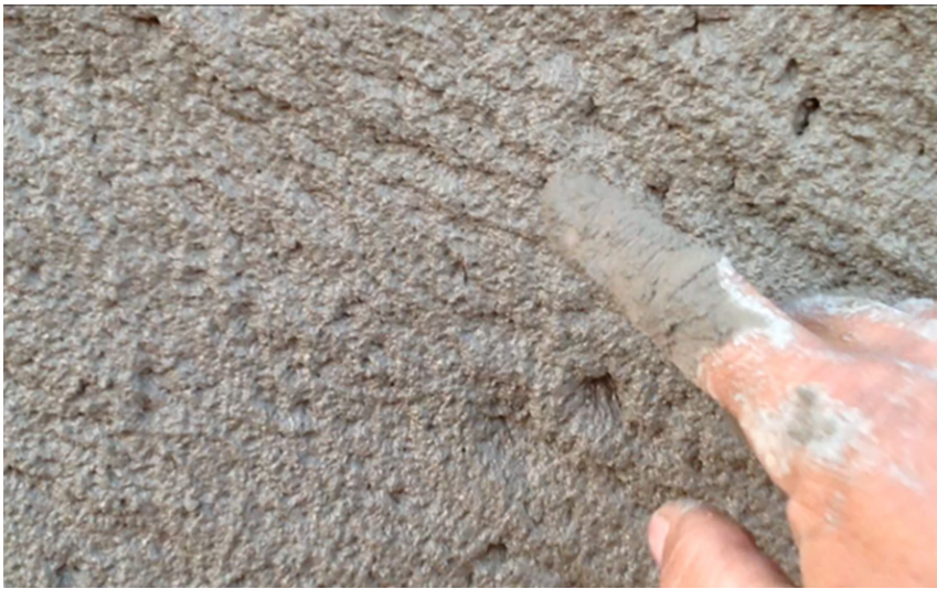
Fig. 9. Freshly applied materials with few visible aggregates at the surface is the visual indicator of a well-chosen slump.
