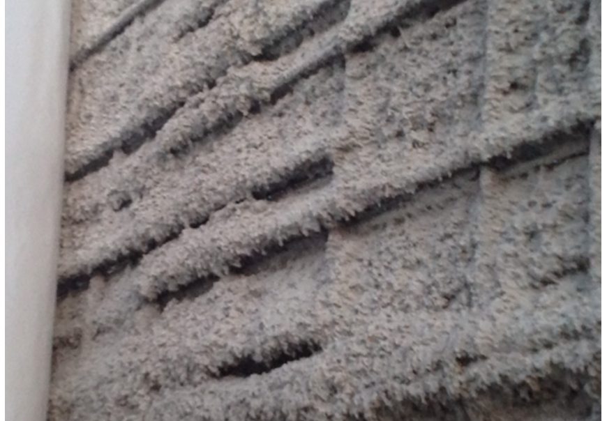
Fig. 5. Visual evidence of buildup on the reinforcement was ignored by the nozzle man. Note the massive voids that have formed behind the bars.
