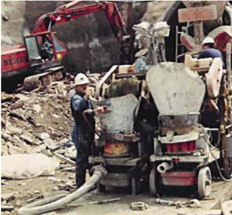
The introduction of the Rotary Gun in 1957 paved the way for large aggregate and high-volume shotcrete
