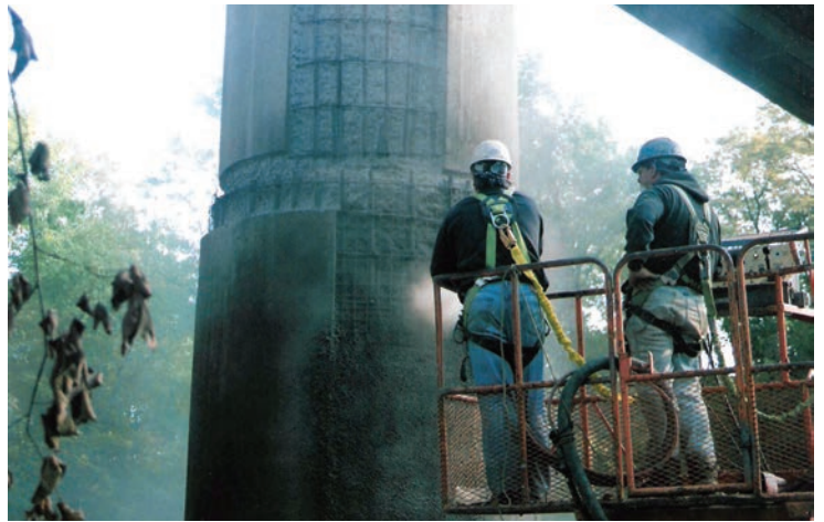
With good surface preparation and gunning practices, shotcrete provides an excellent bond to the existing substrate
