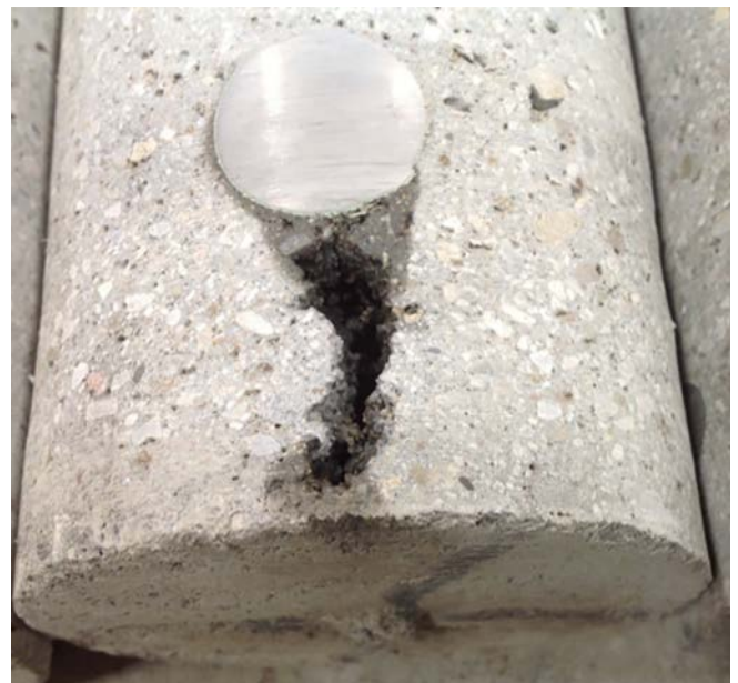
Fig. 2: This core specimen's major flaw is evidence of inadequate flow during placement.
