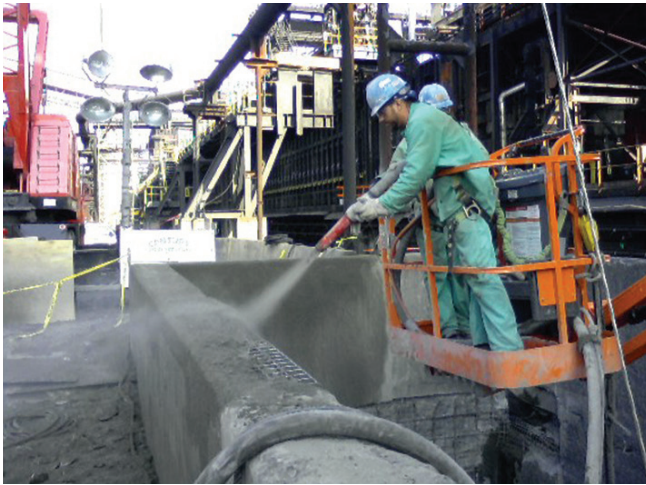
The top of this industrial sump wall is gunned in place using dry-process shotcrete. The shotcrete process provides an excellent natural bond to the substrate without using bonding compounds. In many cases, bonding compounds are detrimental to achieving a good bond with shotcrete
