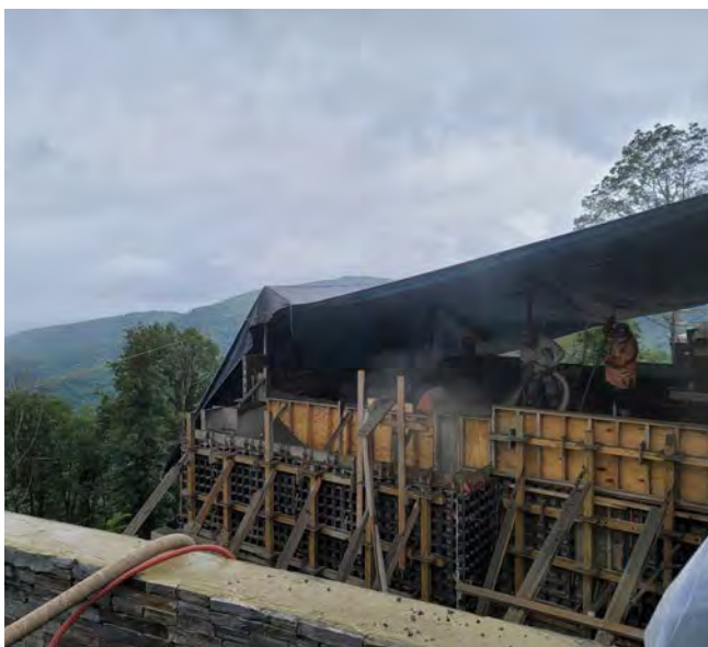
Fig. 3: Rain protection with a tarp. Nozzleman with an air lance operator at his side, keeping the adjacent material clean. Complex forming
