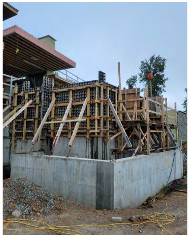
Fig. 5: Pour in place catch basin and foundation walls with forming above for shotcrete placed walls and catch basin floor
