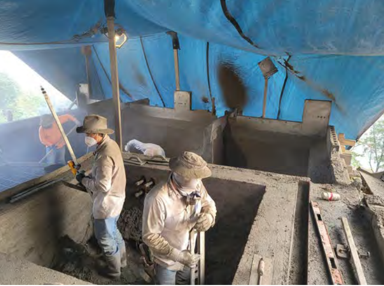
Fig. 6: Finishers working in spa under rain and shade tarp. Upside down boots keep tarp from punching through
