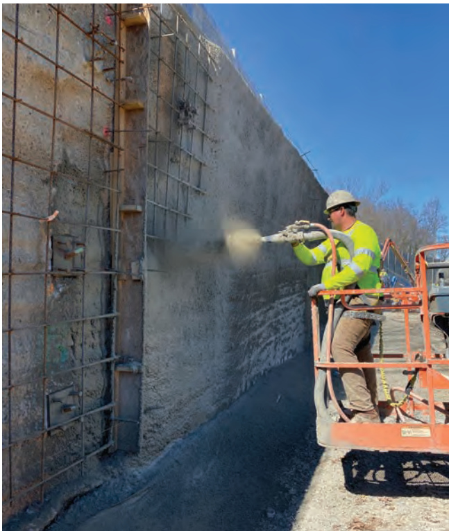
Shotcrete nozzle men worked primarily from manlifts, shooting up to 70 cubic yards of material in a single day
