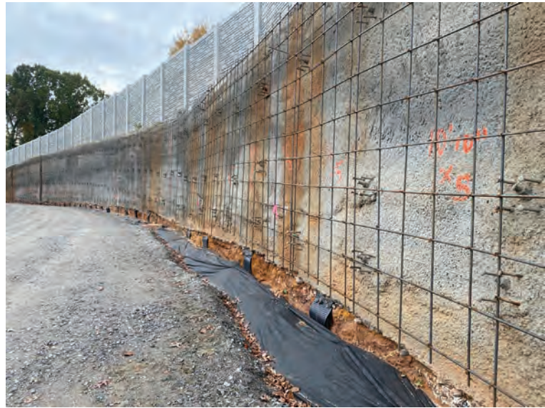
Once the soil nail wall was constructed, several layers of shotcrete were placed in front of it prior to carving the ashlar finish into the final two-inch layer
