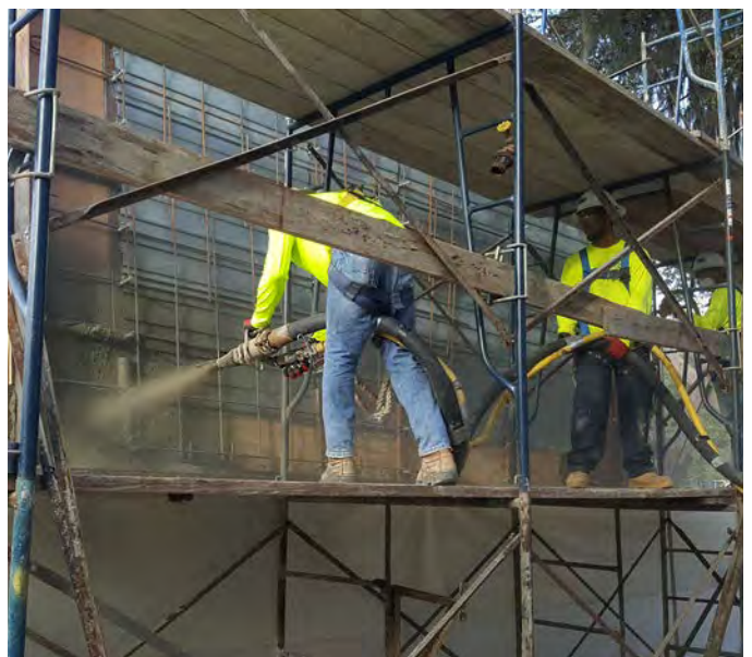
Fig. 5: Mock-up for alternative method of formwork (CROM Project Services Facility Gainesville, FL)
