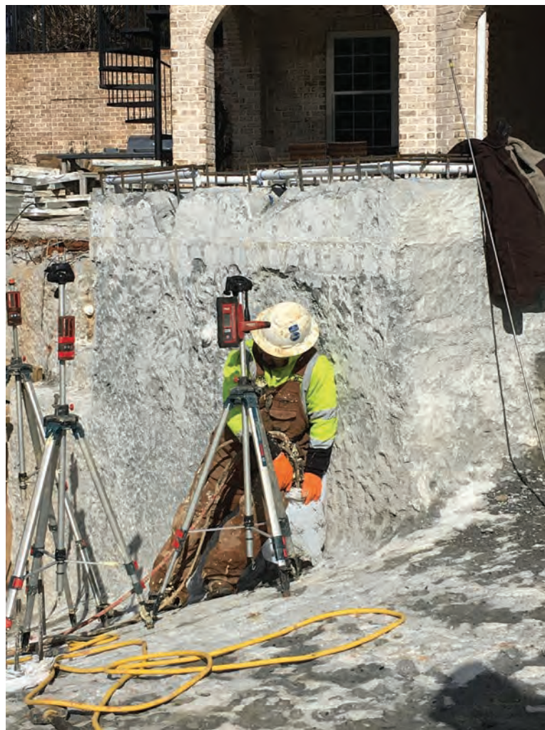
UMA deployed laser measuring devices capable of measuring tolerances within 1/16 of an inch to ensure that no lifting or shotcrete damage occurred.
