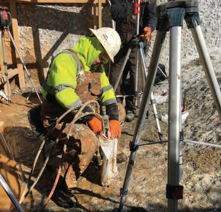
HDPR was injected by performing a series of Deep Injections (DIs) at increments of 3 ft below the bottom of the pool to a final depth of 9 ft.
