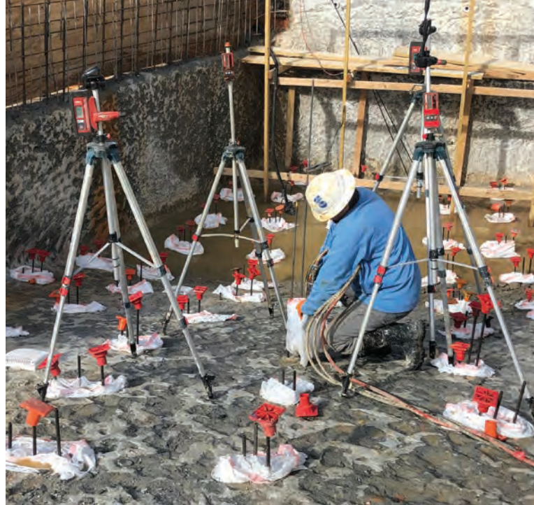
The settlement was easily corrected, and voids were filled without the need to rip out and replace the valuable shotcrete.
