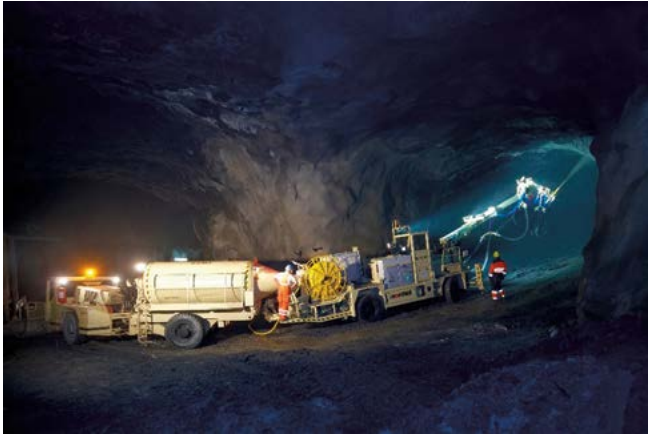
Fig. 6: Typical setup showing concrete hauler (left) feeding concrete pump of mechanized sprayer (right).
