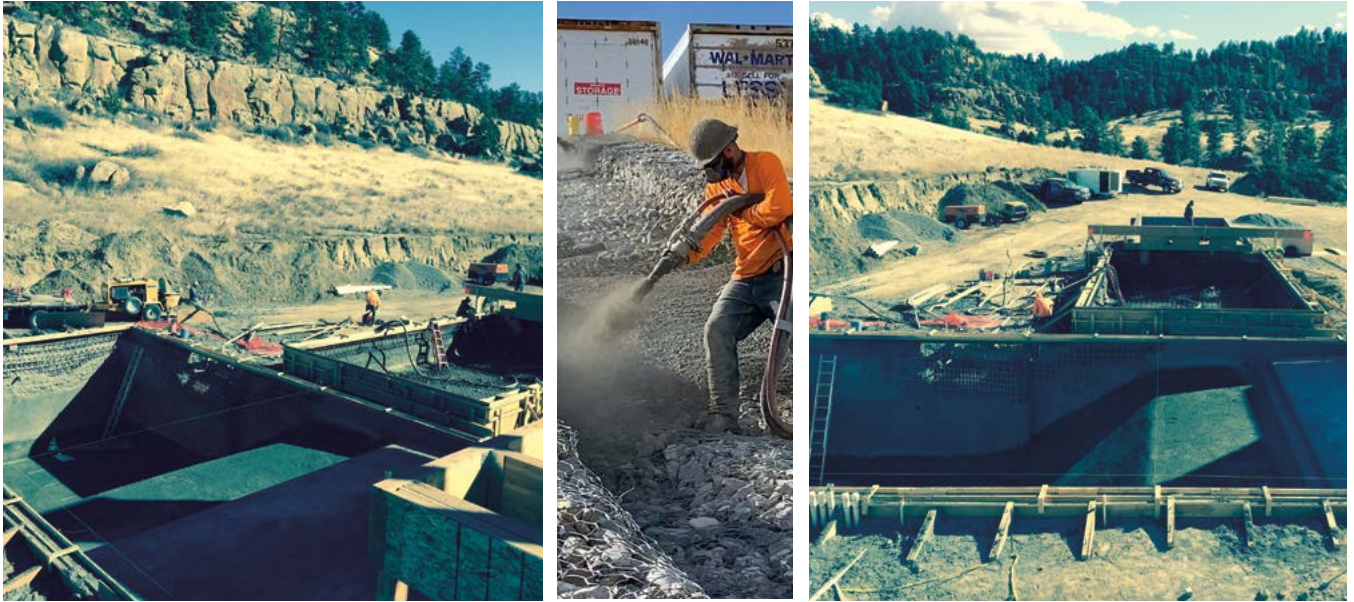
Fig. 3: Project with Separate Sections Shot Simultaneously; Fig. 4: Two Wet-Mix Nozzles – One Pump; Fig. 5: More Flexibility with Two Nozzles
