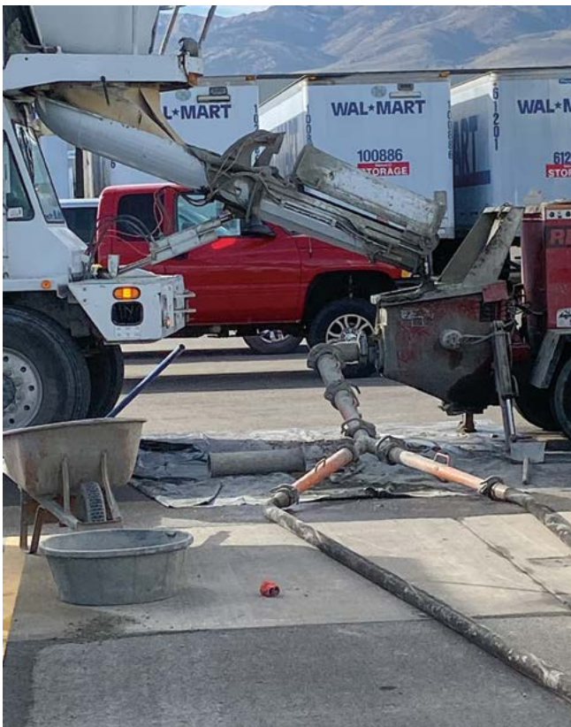
Fig. 6: Delivery Line Splitter on Reducer from Pump
