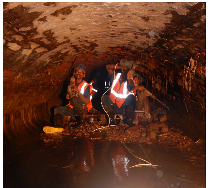
Fig. 4: Root penetration through masonry lining
