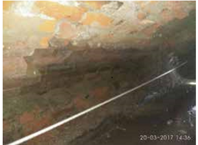
Fig. 2: Delamination and spalling of brick lining
