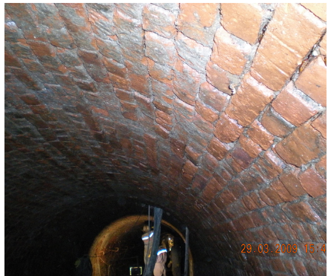
Fig. 3: Erosion of mortar joints
