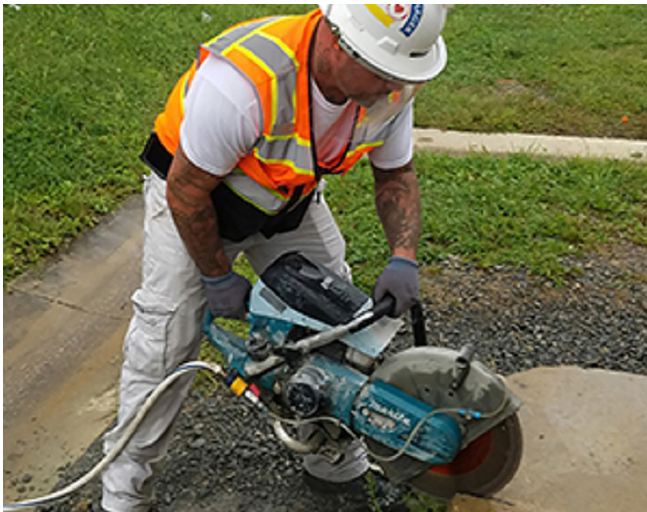
Figure 1: Using water with a cutoff saw when cutting materials that contain crystalline silica substantially reduces the amount of dust created during these operations.
