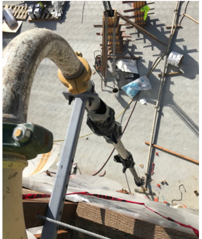
Fig. 1: Long vertical run of shotcrete line, "a shotcrete standpipe"
