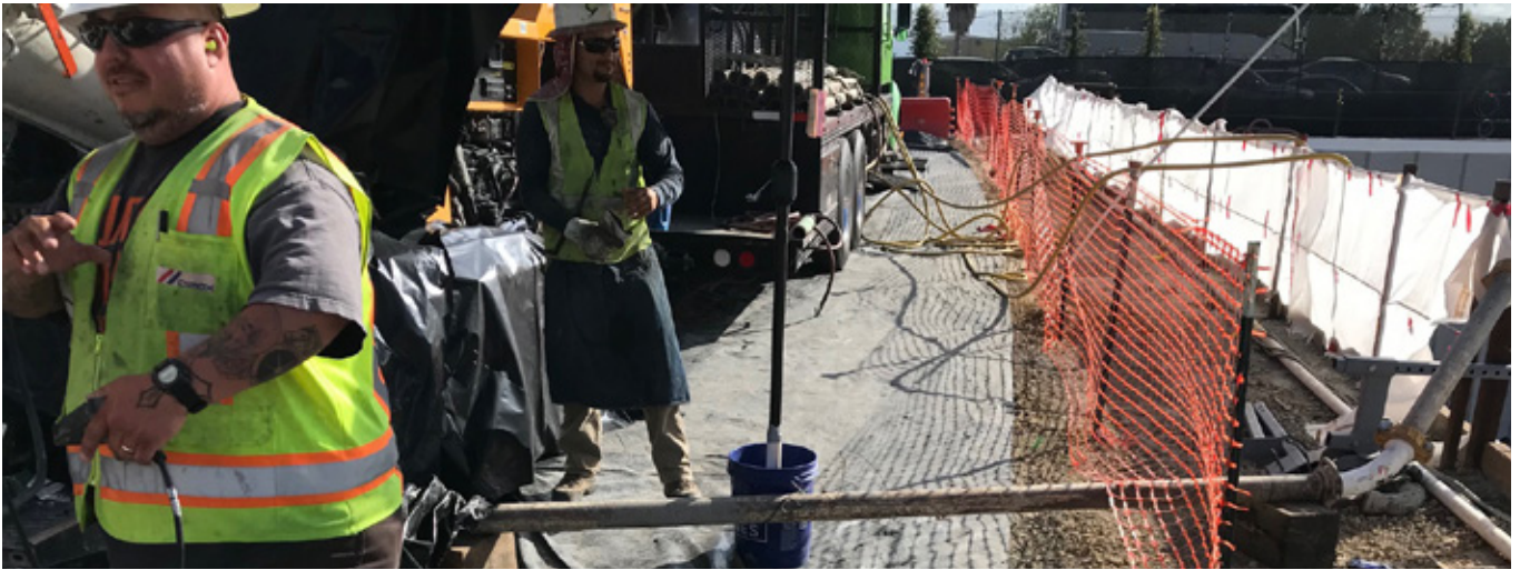
Fig. 2: Steel delivery line exiting pump
