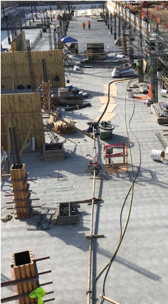
Fig. 6: Steel line transitioning into rubber hose for final discharge
