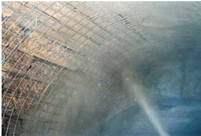
The dry-process shotcrete in this tunnel reline is gunned overhead to the full desired depth without layers
