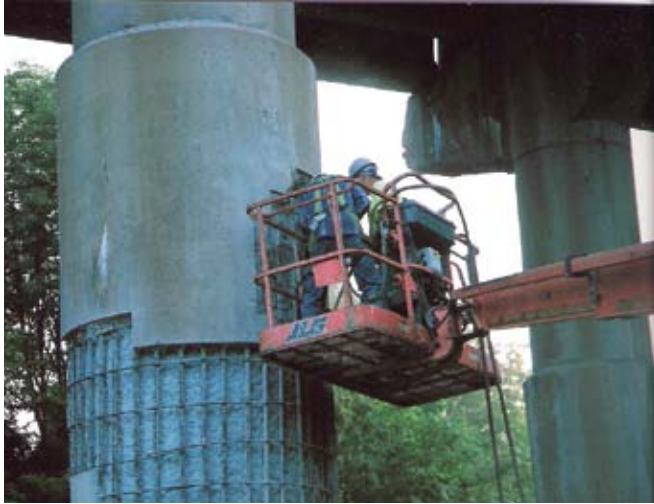
The deteriorated concrete on this bridge pier is removed to behind the first layer of reinforcing bar to allow the shotcrete to fully encapsulate the reinforcing bar
