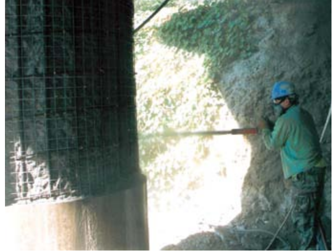
The shotcrete placement on this bridge pier is gunned to the full depth in one continuous pass. It is better to avoid gunning in layers whenever possible
