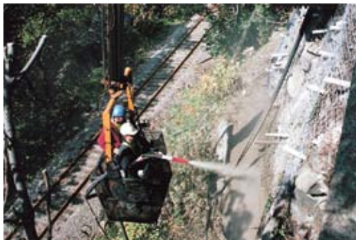
On this slope protection project, the dry-process shotcrete material is gunned to the full necessary depth in one pass
