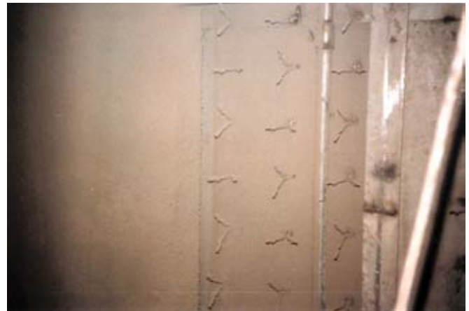
In this power plant ash hopper, the refractory, on the left, is gunned to the full 9 in. (229 mm) depth in one application. The ungunned area with the "V"-type refractory anchors is to the right
