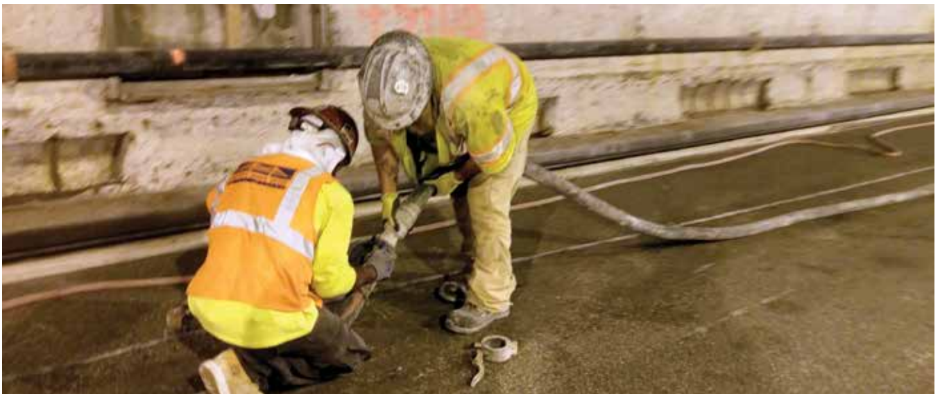
Fig. 7: Cruz's collaborative nature helps to expedite workflow, delivering projects on time and within budget (Photo courtesy of Cruz)
