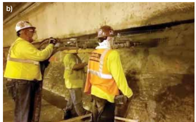
Fig. 6(a) and (b): A prepared fireline sits within the walls of the QMT (top). Cruz's device to reduce the stress of employees while ramping up productivity (lower) (Photo courtesy of Cruz)
