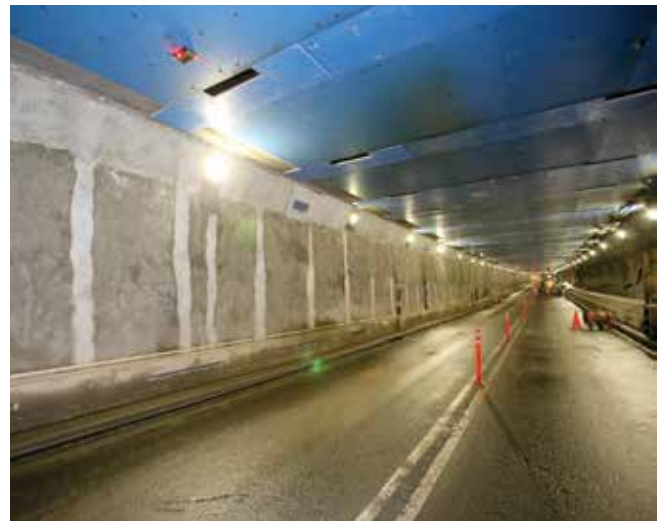
Fig. 4: Post-construction image of shotcrete, light trenches have been repaired (top left), the drainage chases have been chipped out and replaced (vertical lines) and ceiling has been patched and encased with fireproof panels (Photo courtesy of Judlau)
