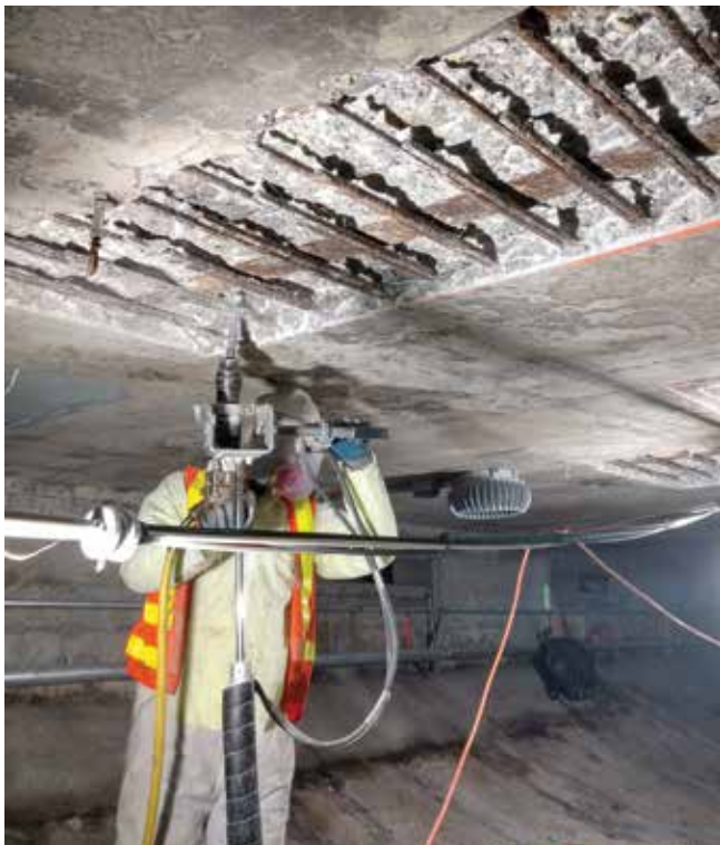
Fig. 5: Working in the air ducts provided for tight work spaces for the entire crew. Cruz devised methods to ease human comfort while working in these situations. Crew chipping away deteriorated concrete (Photo courtesy of Cruz)
