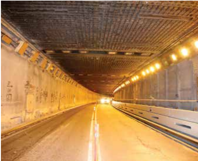
Fig. 2: Preconstruction, highlighting the light trenches ready for wet-mix shotcrete (top left), hollow wall niches (right wall) and exposed ceiling for patch repair (Photo courtesy of Judlau)
