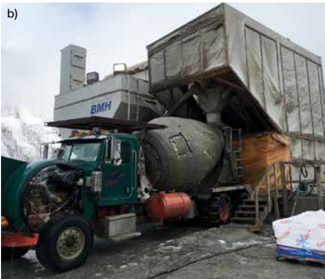
Fig. 2(a) and (b): On-site shotcrete batching; note that the batch plant and concrete truck were insulated for the cold weather
