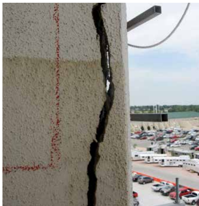
Fig. 2: Crack in monumental concrete column
