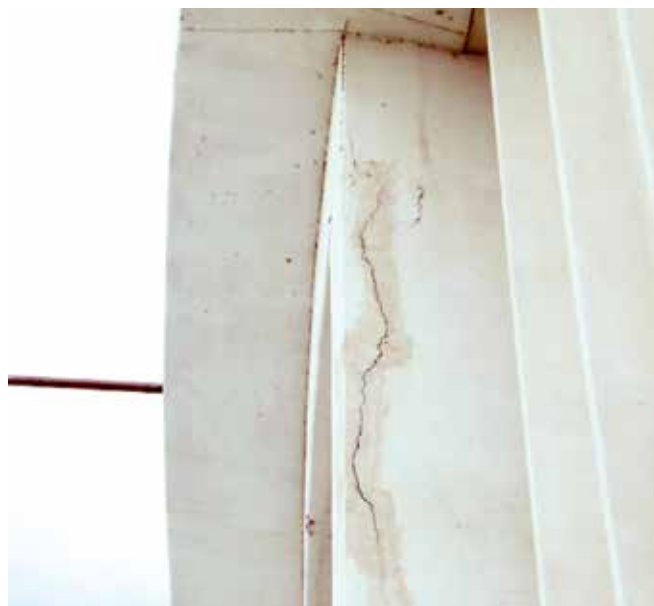
Fig. 1: Cracking in monumental concrete column
