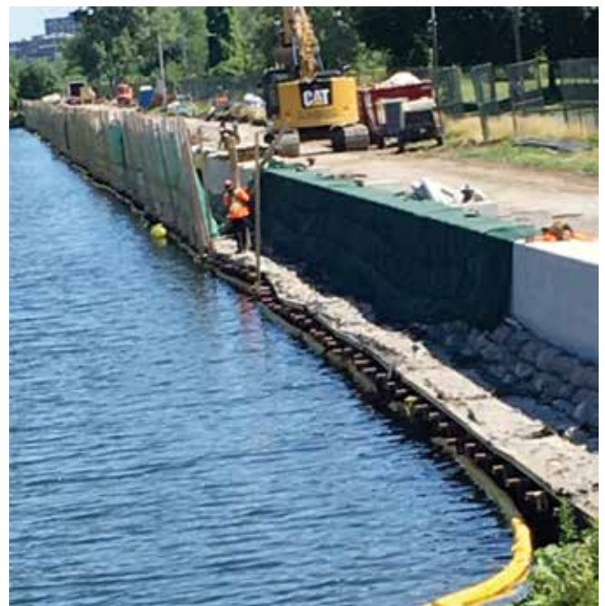
Fig. 3: Protective barrier and floating boom
