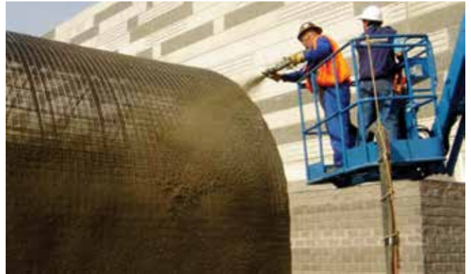
Fig. 7: Wet-mix shotcrete and air hoses secured to the manlift basket (Shotcrete Technology Transfer Expo, Santiago, Chile)
