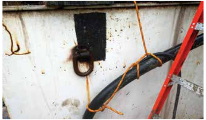
Fig. 6: Wet-mix shotcrete and accelerator hose secured to the work platform (GAB Pedestrian Tunnel, Richmond, VA)
