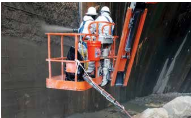
Fig. 5: Close-up of dry-mix shotcrete and water hose secured to the manlift while moving. The rope keeps the hose from pulling out of the basket (Buchanan Dam, Llano County, TX)
