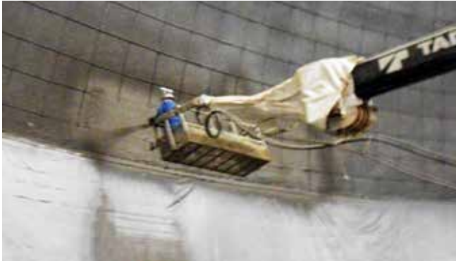
Fig. 3: Wet-mix shotcrete hose secured to the boom and basket while shooting a concrete dome (Rain CII, Gramercy, LA)
