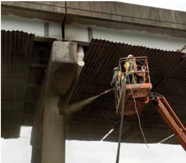
Fig. 8: Gunning of prepackaged material on bridge pier. We were required to repair one side of the piers at a time
