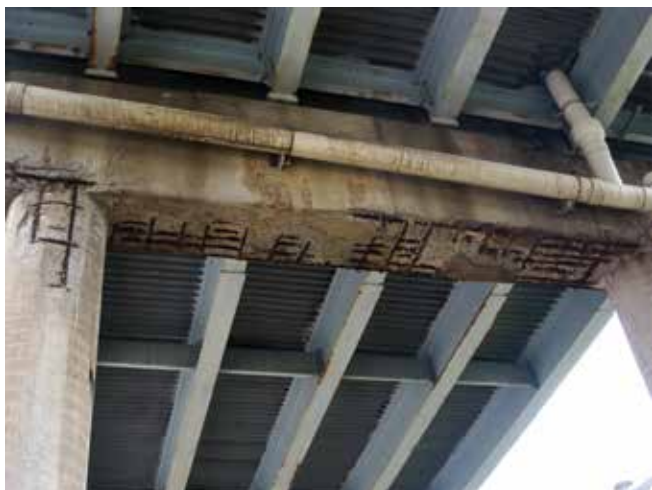
Fig. 2: All but one of the bridge piers had deterioration where repairs were necessary
