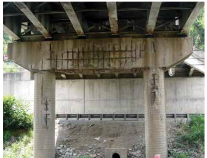
Fig. 5: Because of concerns about the condition of this pier the repairs were performed in four phases
