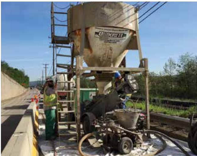
Fig. 7: Material hopper, predampener, and continuous-feed rotary gun setup for gunning prepackaged shotcrete repair mortar
