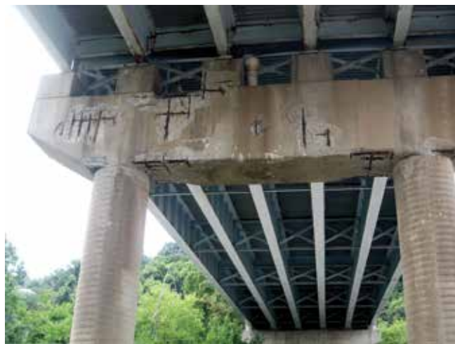
Fig. 3: When reinforcing bars close to the concrete surface corroded, the expansion of the rust spalled concrete off the rusted bars
