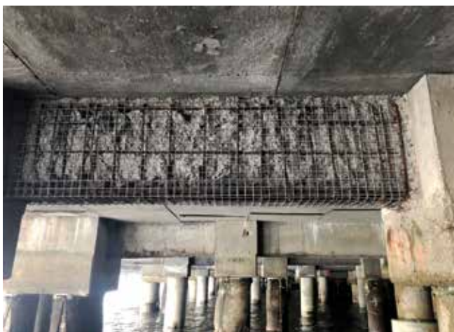
Fig. 2: A Type 3 repair with preparation completed. The repair is awaiting the application of shotcrete
