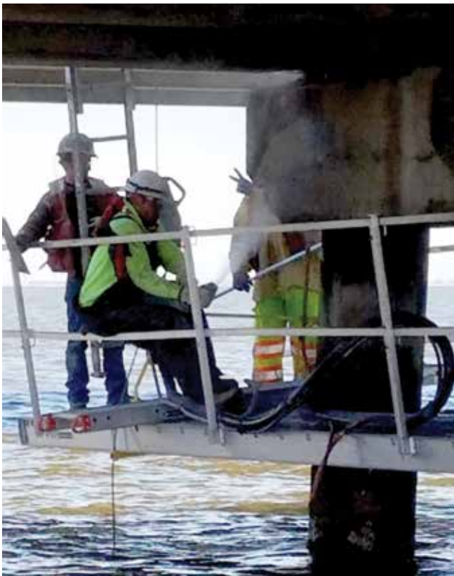
Fig. 3: Nozzlemen shooting back damaged bent cap
