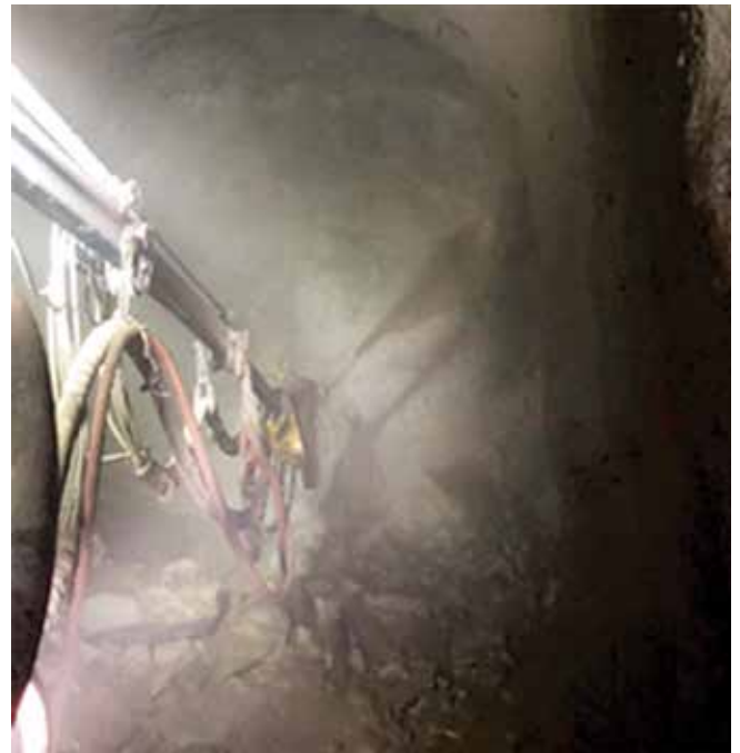
Fig. 2: The admixtures play an important role in the production of this underground shotcrete placement
