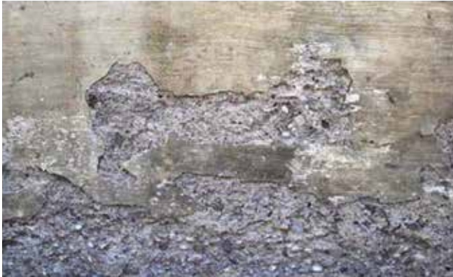
Fig. 6: Severe surface scaling on the concrete
