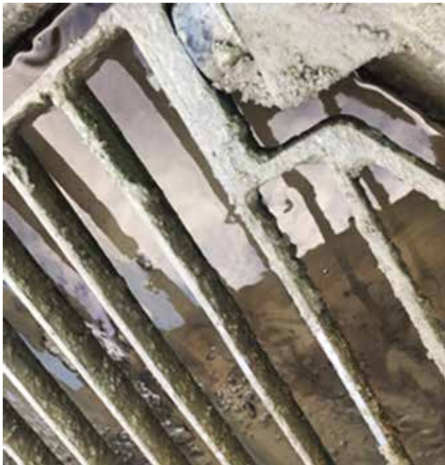
Fig. 1: Obviously too much water on top of the concrete in the hopper
